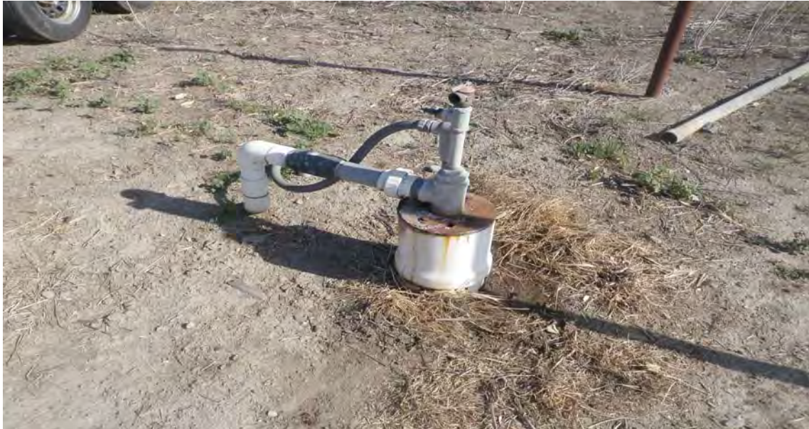
Photo 1: Well #1 with no well-pad.
