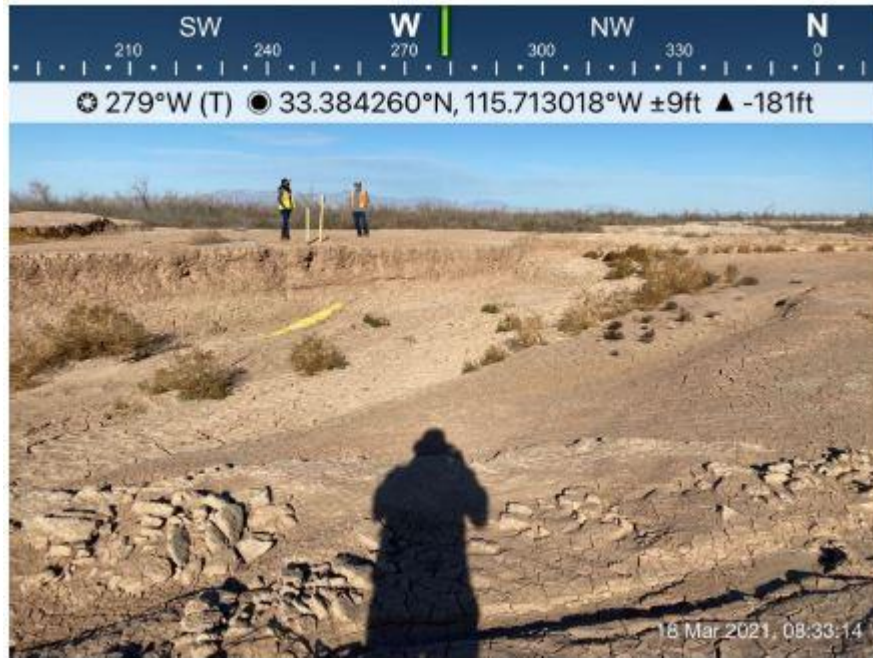
Figure 6 Photograph looking west towards the exposed pipeline and the Project work area.
