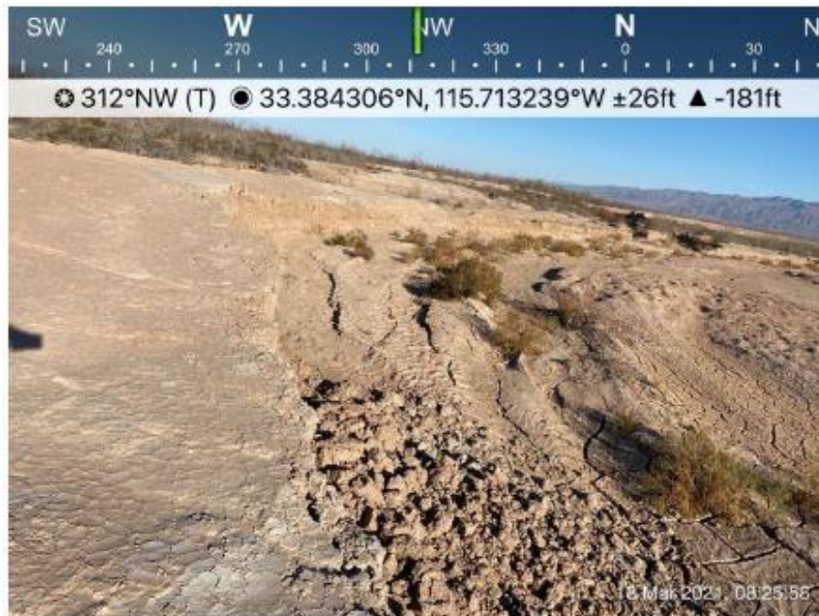
Figure 5 Photograph looking northwest (upstream) from the exposed pipeline, showing dried mudflat areas and channel.
