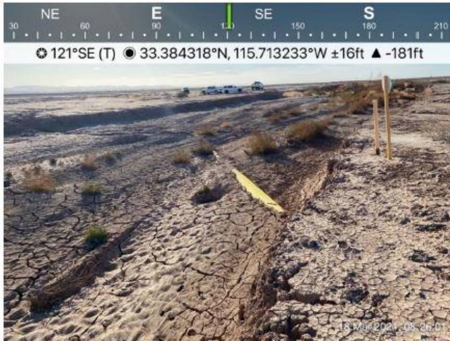
Figure 4 Photograph looking southeast (downstream) towards the exposed pipeline within the dried mud channel.
