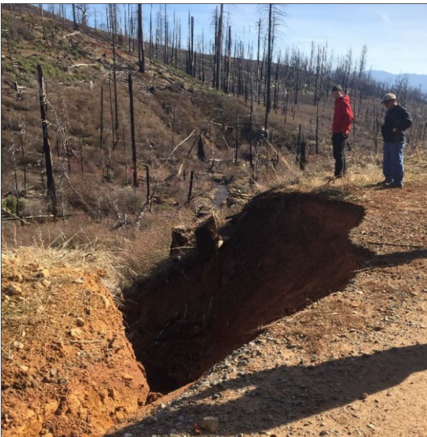
Figure 5.3 - Timber access road fill slope collapse from intercepted surface water conveyance.
