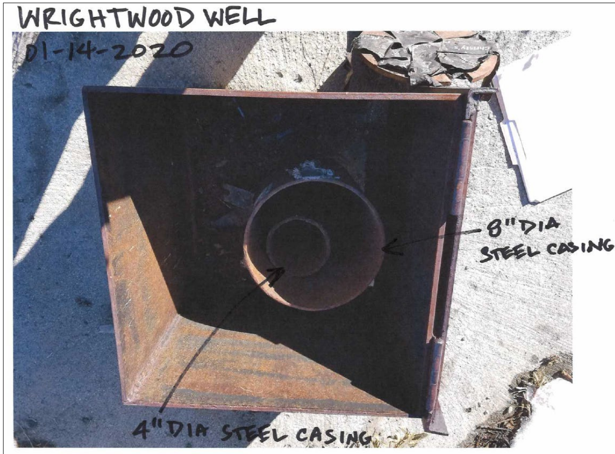
Figure 13.5 - Former San Bernardino County Services Area (CSA) 56 monitoring well. There is no secured cover. The steel casing is not secured and locked and the steel box cover is not secured to.
