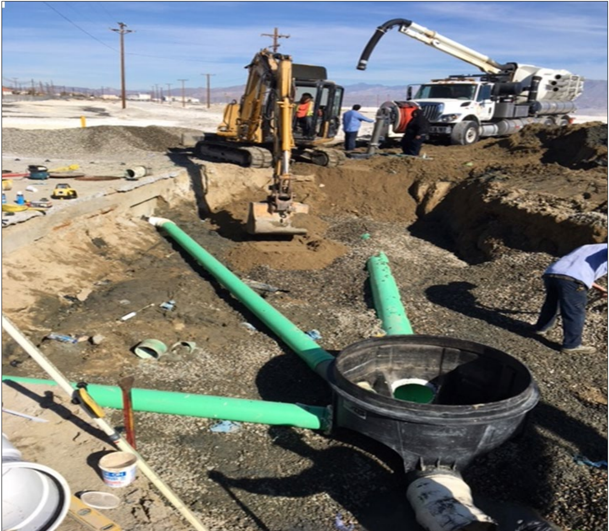
Figure 9.5 - Project to restore flow in the effluent outfall pipeline after earthquake changed infrastructure elevations.
