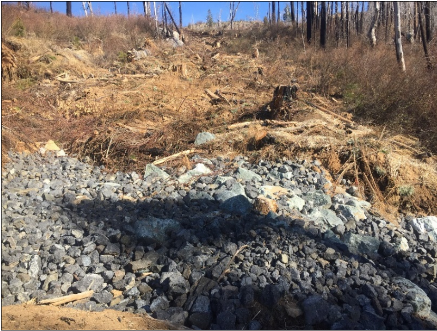
Figure 5.4 - Creek hillside damaged from timber harvesting equipment. Rock fill was used to prevent sediment delivery to the creek below.
