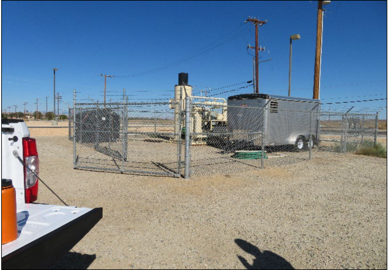
Photo 3.1: View of the air sparge (AS)/soil vapor extraction (SVE) system at Site 297. The SVE system (beige system in background) was upgraded with a new Mako Industries Inc. (Mako) thermal/catalytic oxidizer SVE system in June 2021. This replaced the repurposed Baker Furnace SVE system that was installed onsite in 2019.
