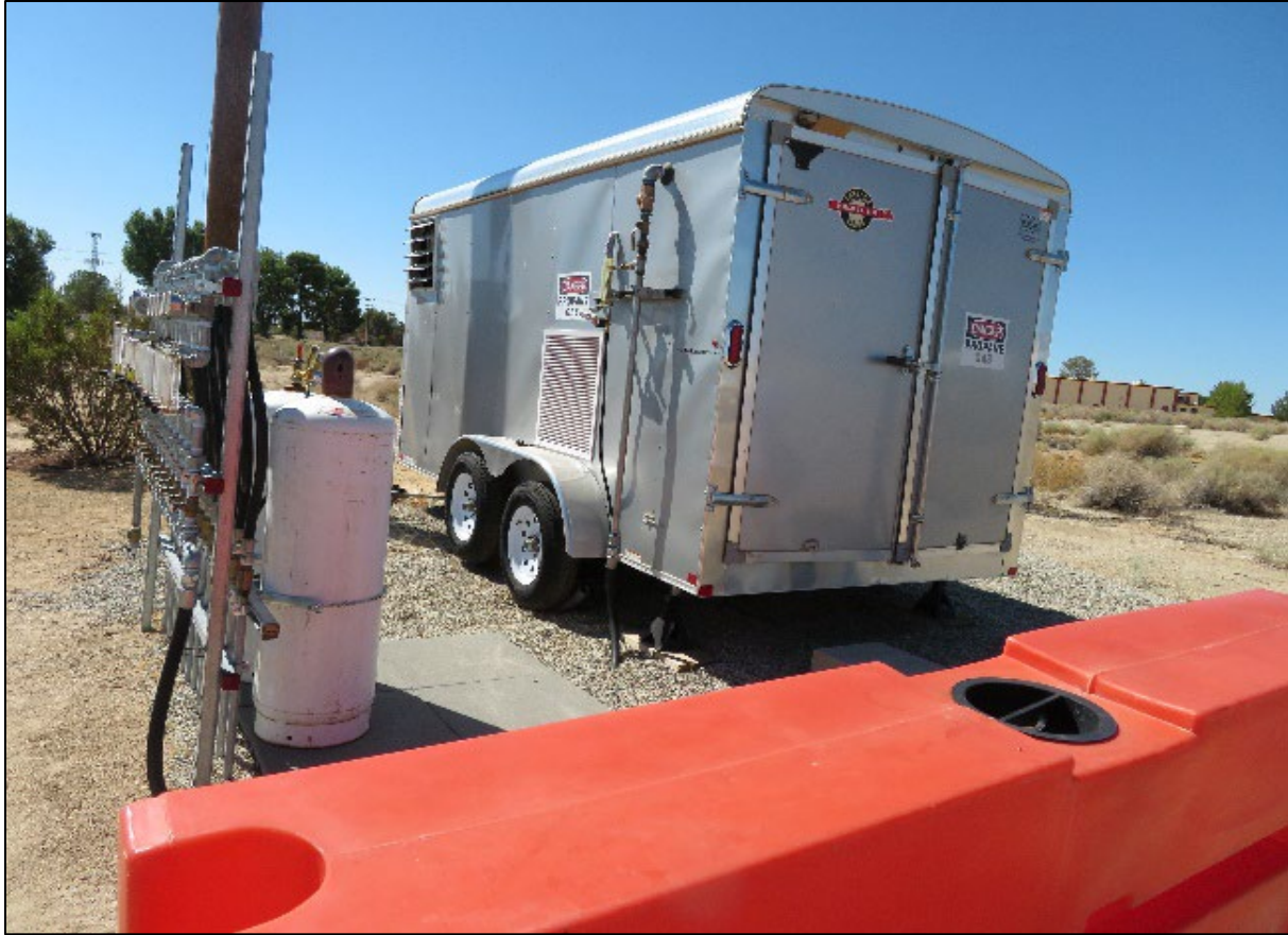
Photo 3.2: View of the upgraded BioSparging system at Site 298. Air compressor was upgraded/replaced (inside of trailer). Several flow regulators were also upgraded (seen on left side of photo) so that more air can be delivered to the subsurface.
