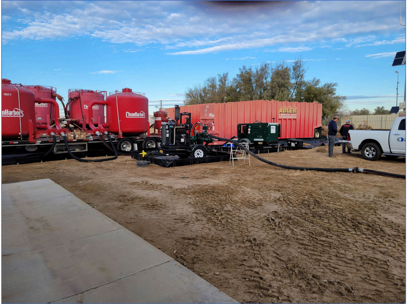
Photo 5.1 – Hose leading to black pump (center), treatment cannisters (bright red on left), and to equalization tanks (light red on right).
