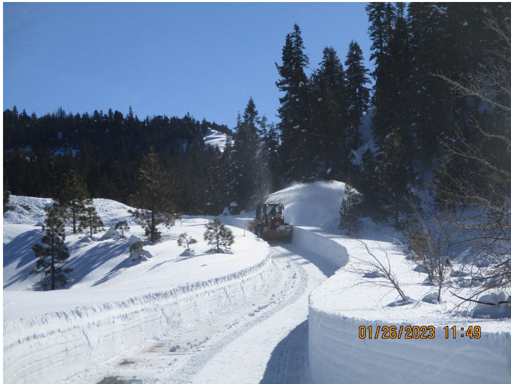
Photo 1 – January 26, 2023, Initial snow removal activities approaching the Pond 1 area. Snow depth approximately 4-5 feet in this area.
