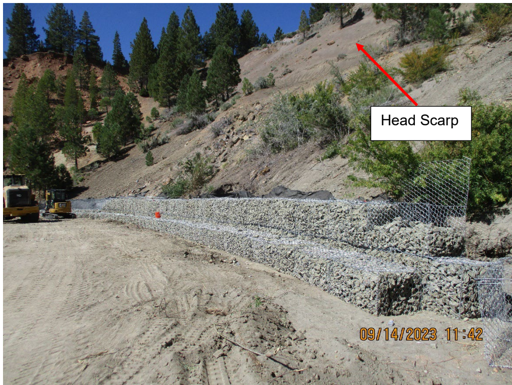
Photo 24 – September 14, 2023, Installation of rock filled gabion baskets to buttress the toe of the Pit Slump.
