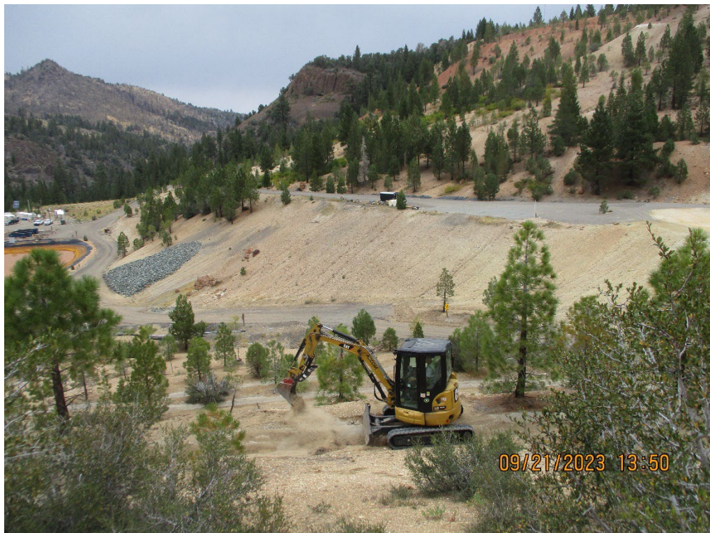
Photo 16 – September 21, 2023, Removal of accumulated sediment from the stormwater conveyances on the Pond 2 North berm.
