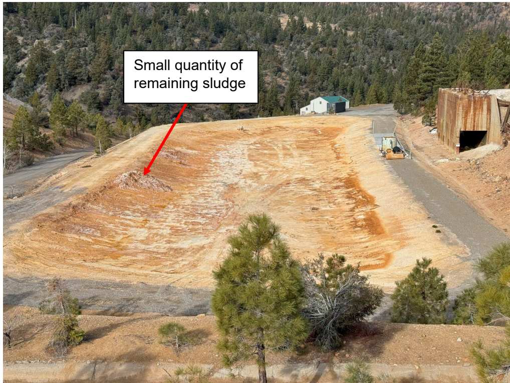
Photo 15 – November 30, 2023, Pond 3 after the completion of sludge haul activities. A small quantity of sludge (less than half a truck) was left following haul activities and will be hauled next season.
