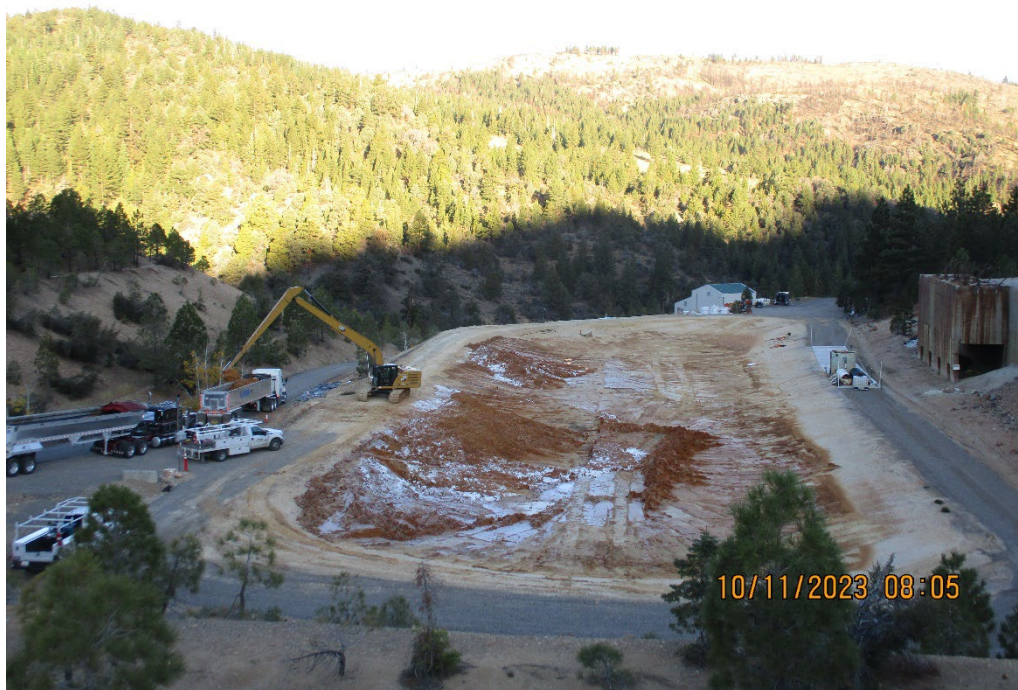
Photo 14 – October 11, 2023, Sludge haul at Pond 3. The white material is Aprumud P100XL, a highly absorbent non-hazardous polymer powder used to absorb water and solidify the sludge for shipment.
