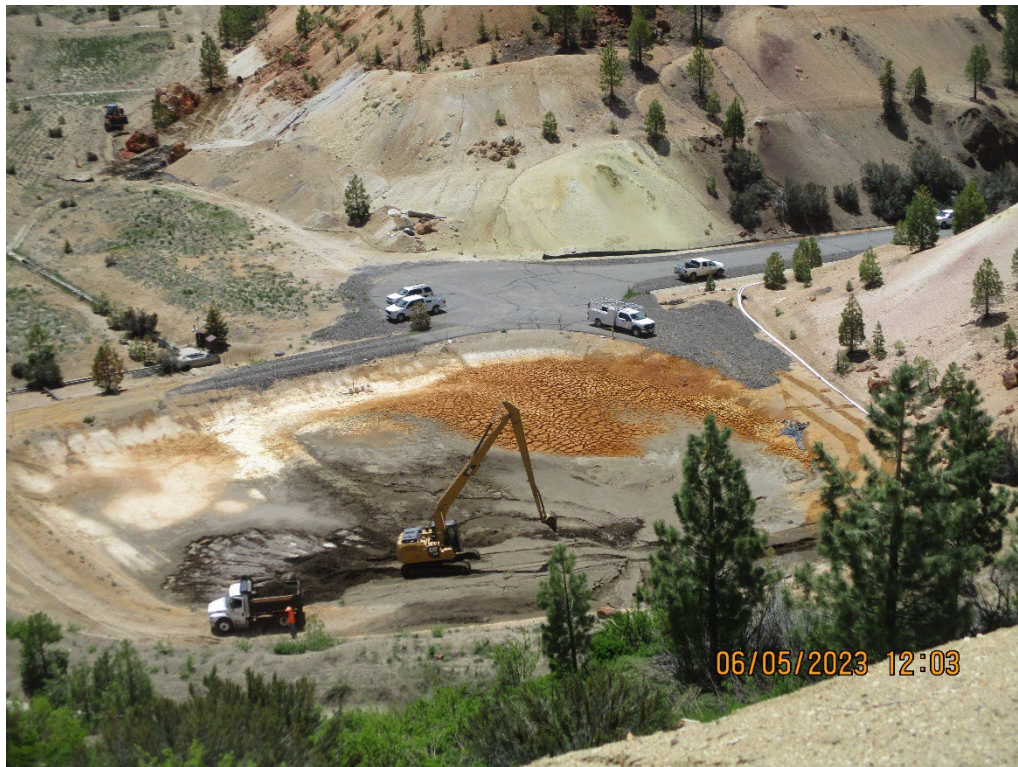
Photo 21 – June 5, 2023, AECOM beginning removal of Pit Slump debris from the Pit Clarifier.
