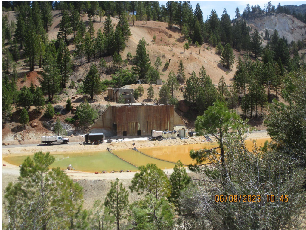
Photo 7 – June 8, 2023, TKT utilizing two turbidity curtains in Pond 3 to improve sludge management and discharge quality.
