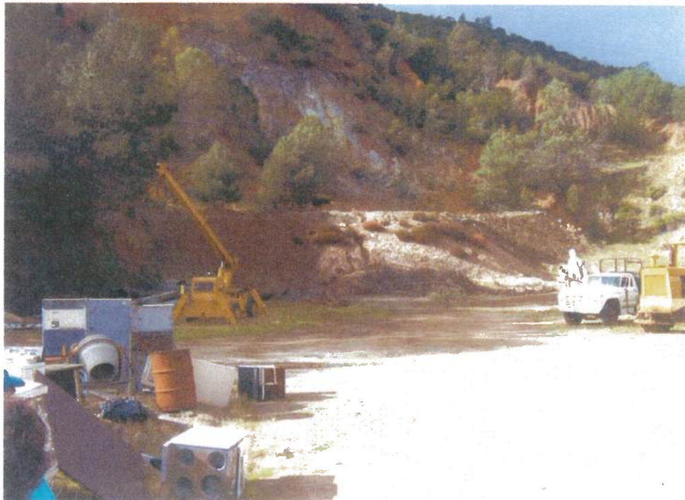
Photograph B-2: Capped area overlying the historic collapsed main mine workings area.
