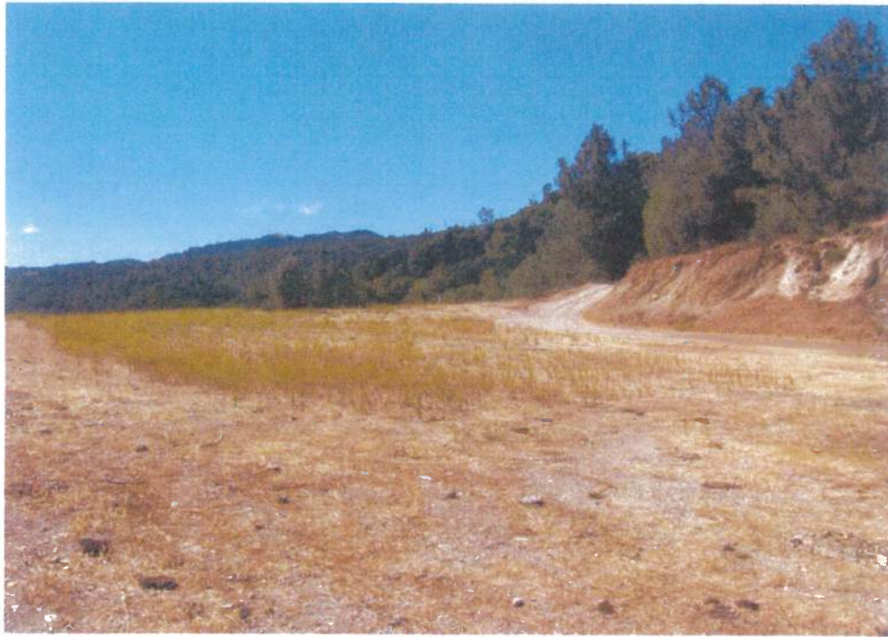
Photograph B-1: Capped area located at the top area of the Bradley tailings piles and waste rock.
