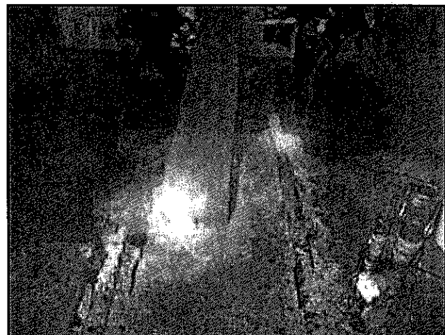
Photo 24. Showing water leaking from the area of the mine seal pooled below the 4-inch shutoff valves.
