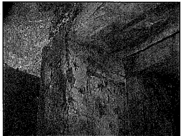
Photo 24. Compressed Rotten Timber.
