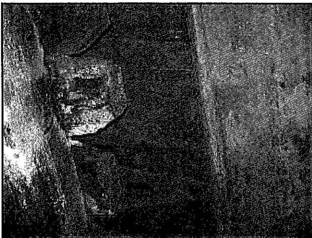
Photo 27. Broken Timber and Crown Bars.
