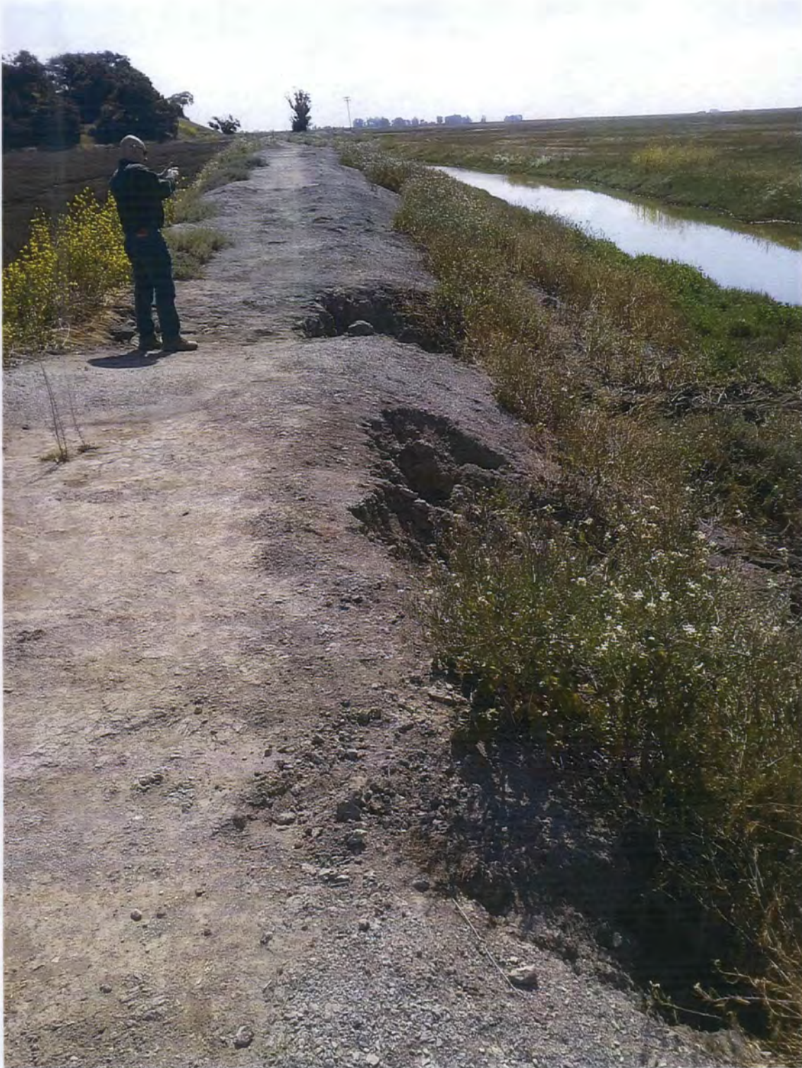
Photo 8: Second Levee Failure Location looking west at eroded backside indicating that water overtopping the levee is causing it to fail.
