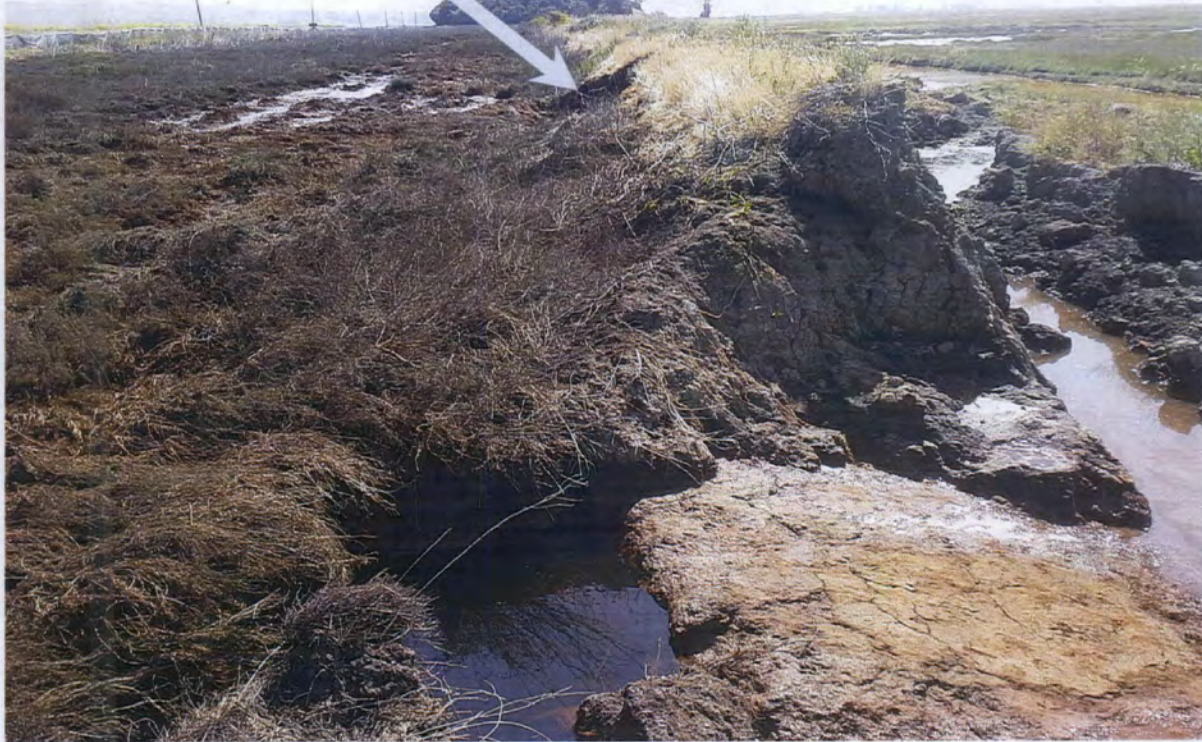
Photo 3: Breach 1 at First Levee Failure Location looking east. Water is discharging from the salt marsh on the left to the channel and seasonal wetlands to the right as it would during high tides.
