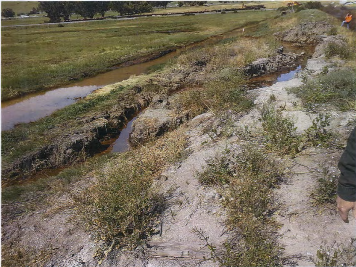
Photo 7: First Levee Failure Location looking west at backside of failed levee (i.e., the side not exposed to the tides).
