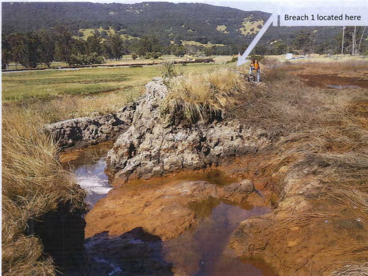
Photo 6: Breach 2 at First Levee Failure Location looking west at discolored water discharging from salt marsh to channel on CDFW property.
