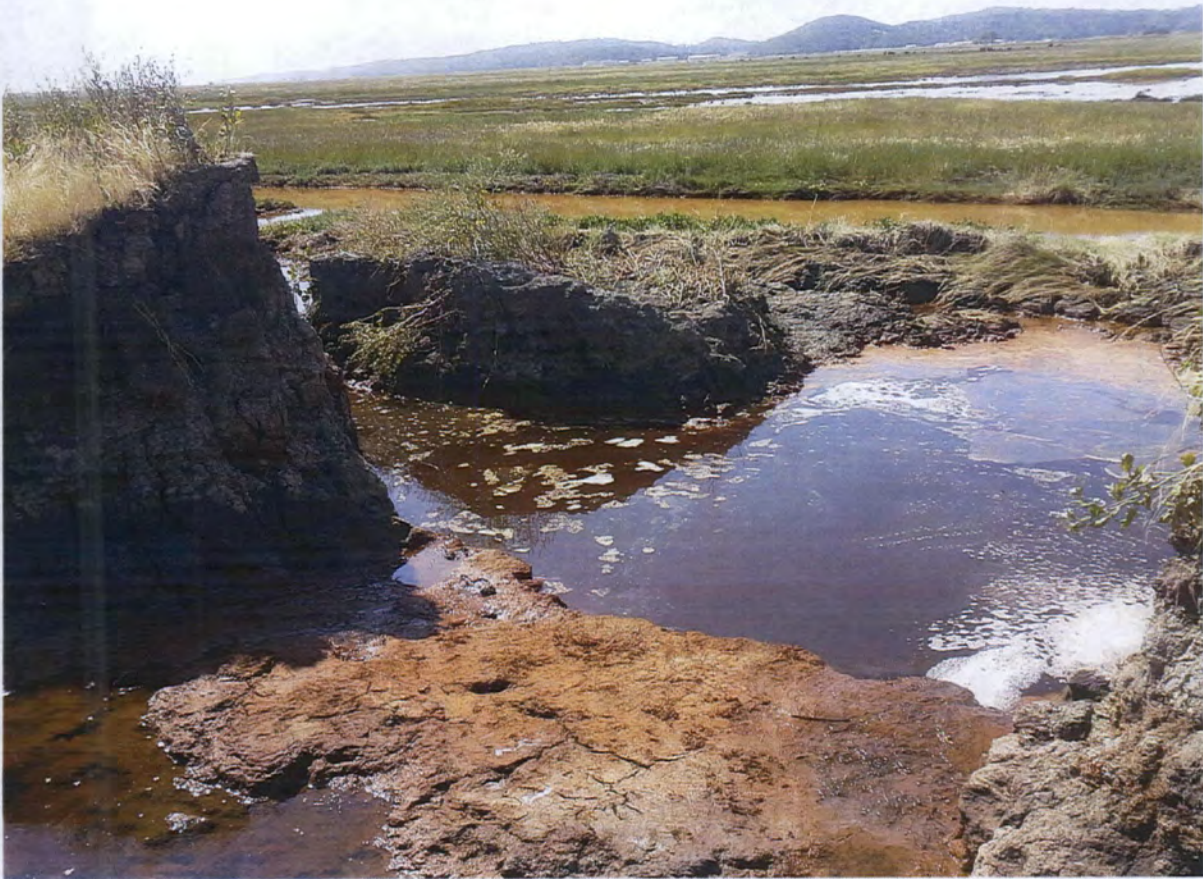
Photo 5: Breach 2 at First Levee Failure Location looking south at discharge of discolored water.
