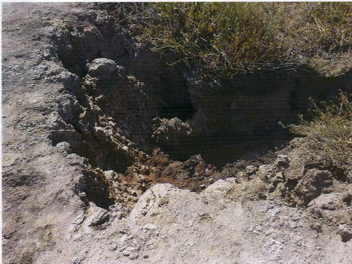
Photo 10: Second Levee Failure Location looking at eroded backside.
