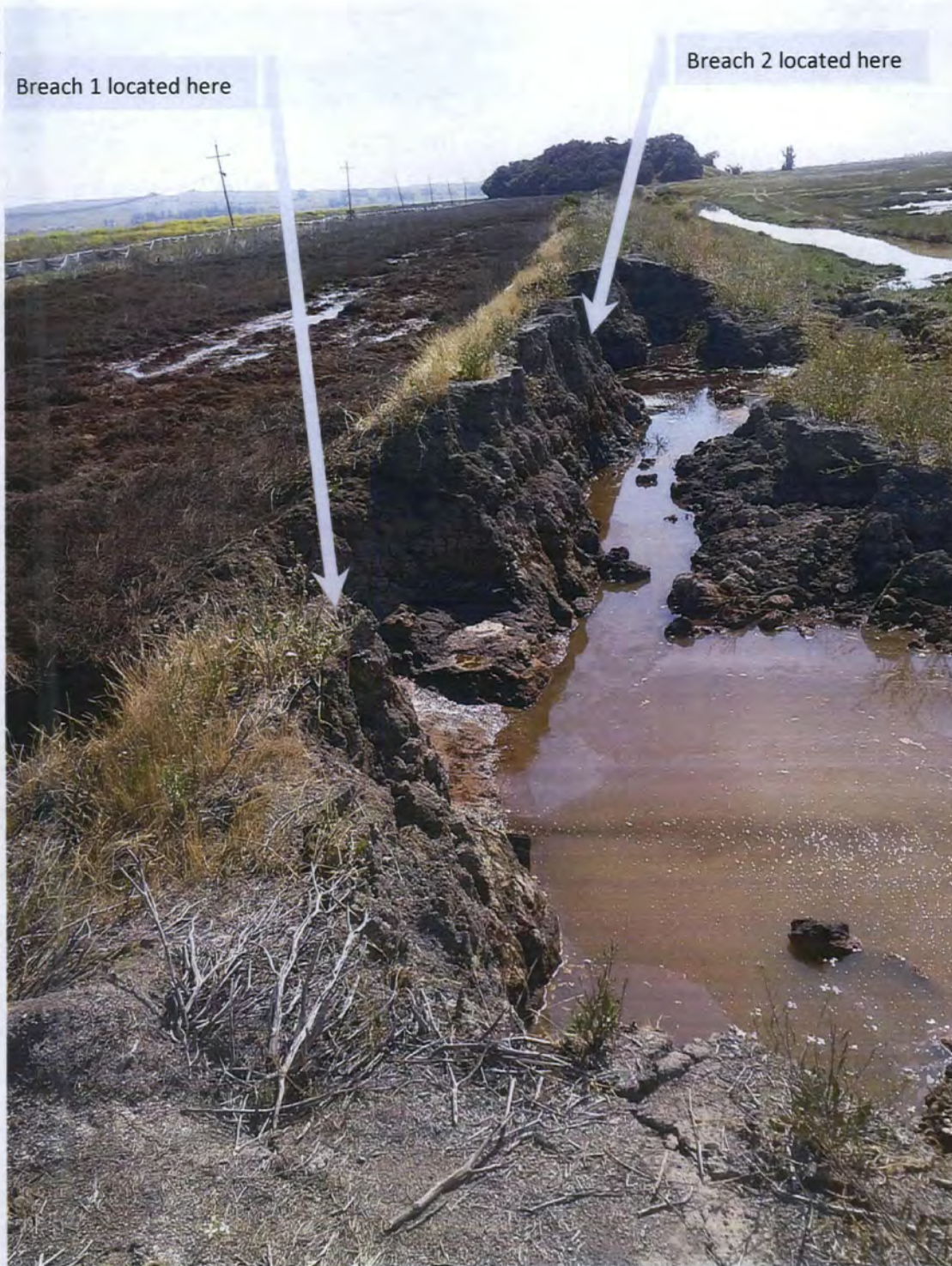
Photo 1: Two breaches at First Levee Failure Location looking east. Power lines to left are located on access road that separates the Mira Monte site owned by SMART from CDFW property, which includes the salt marsh to the left of the levee and the channel and seasonal wetlands to the right of the levee shown in the photo. The condition of the levee separating the two breaches is severely comprised and will likely fail if not addressed before it is exposed to high tides.
