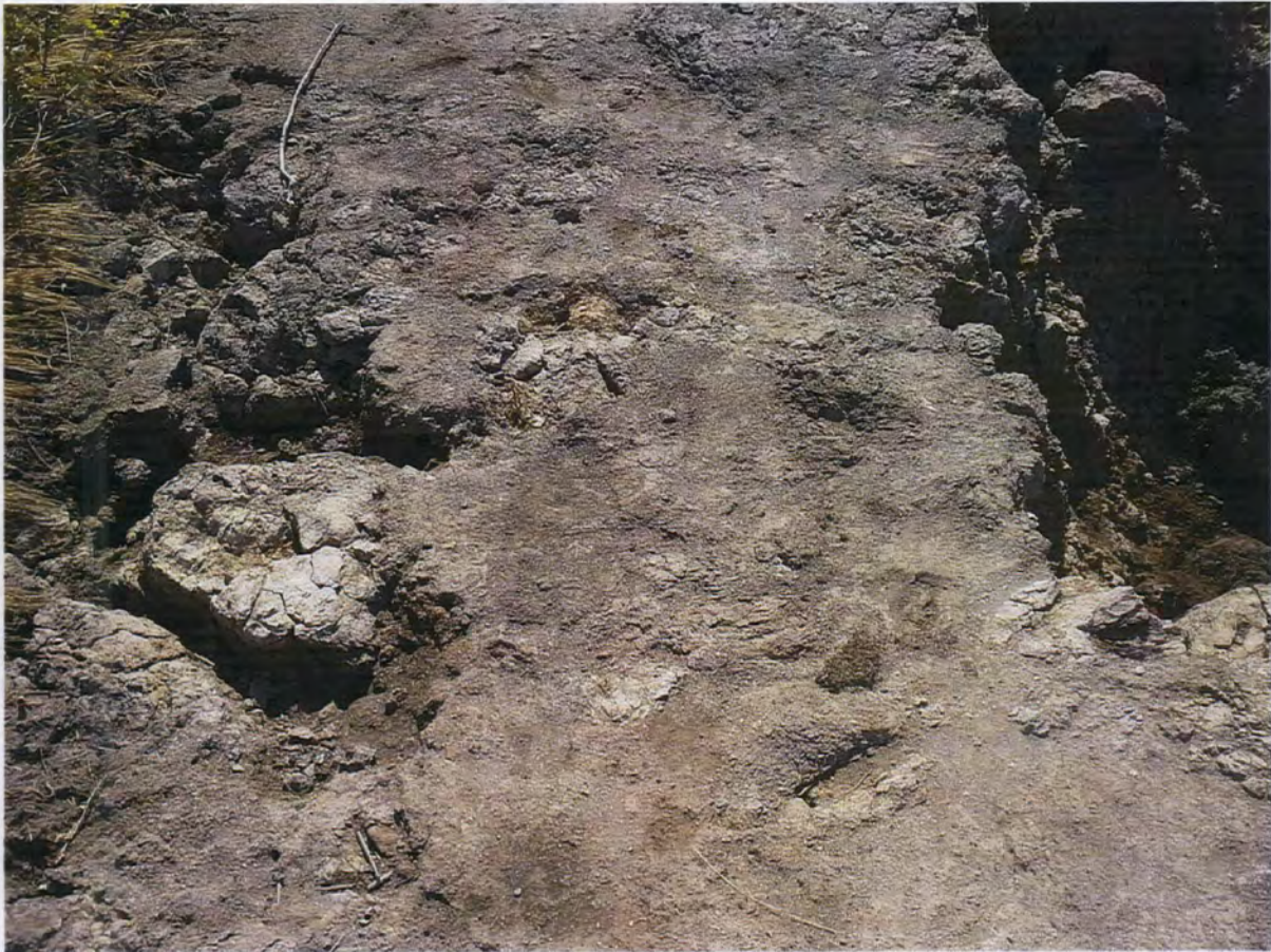
Photo 9: Second Levee Failure Location looking at erosion caused by overtopping of levee.
