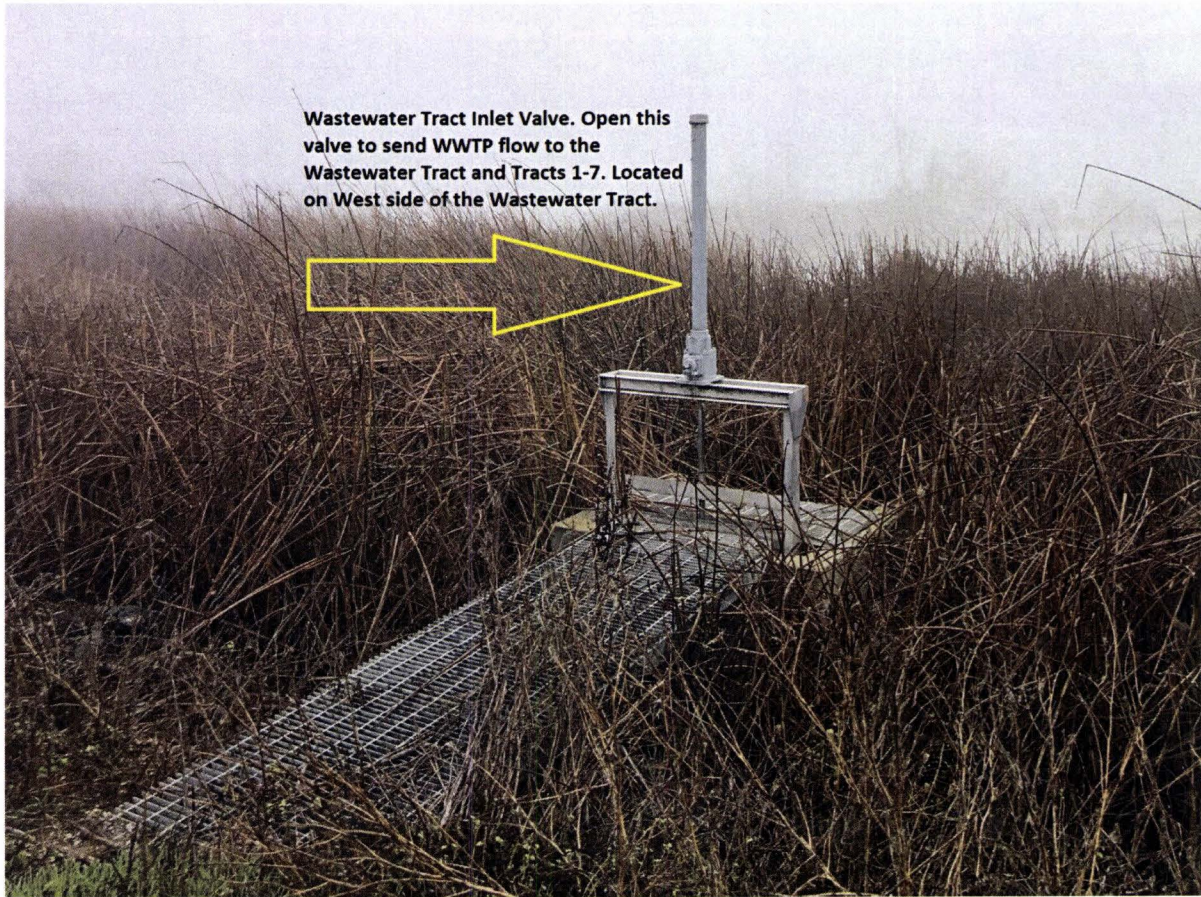
Figure 10: Wetlands Wastewater Tract Inlet 10/3/22
