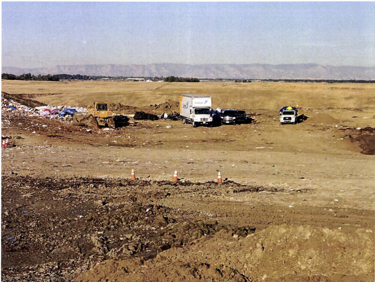
Figure 1: Active disposal area and access roads. Recycled water will be used for dust suppression 10/3/2022
