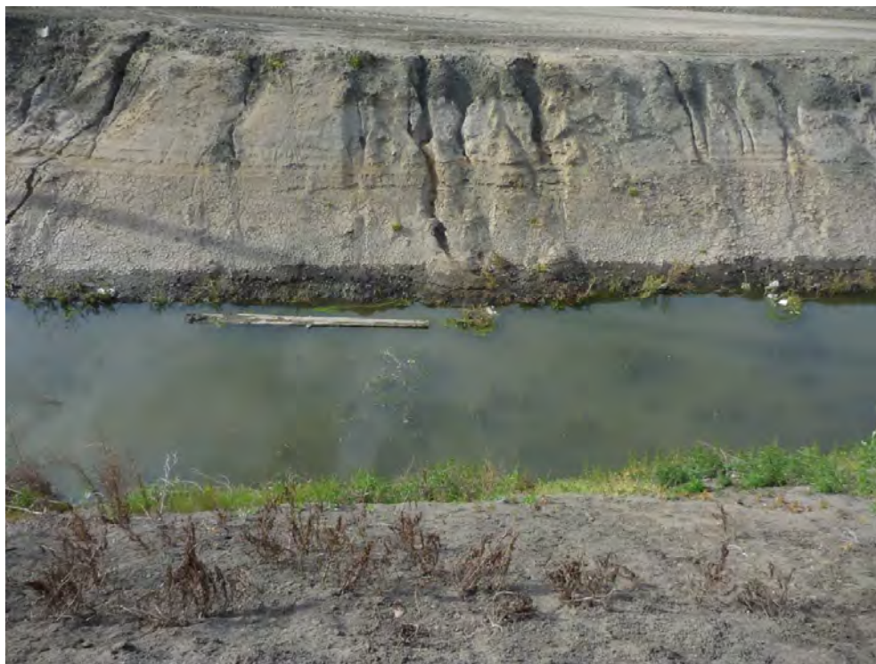
Figure 28. Photo of bank rilling and erosion the Salinas Reclamation Canal upstream of Highway 101. Source (MCWRA, 2015a).
