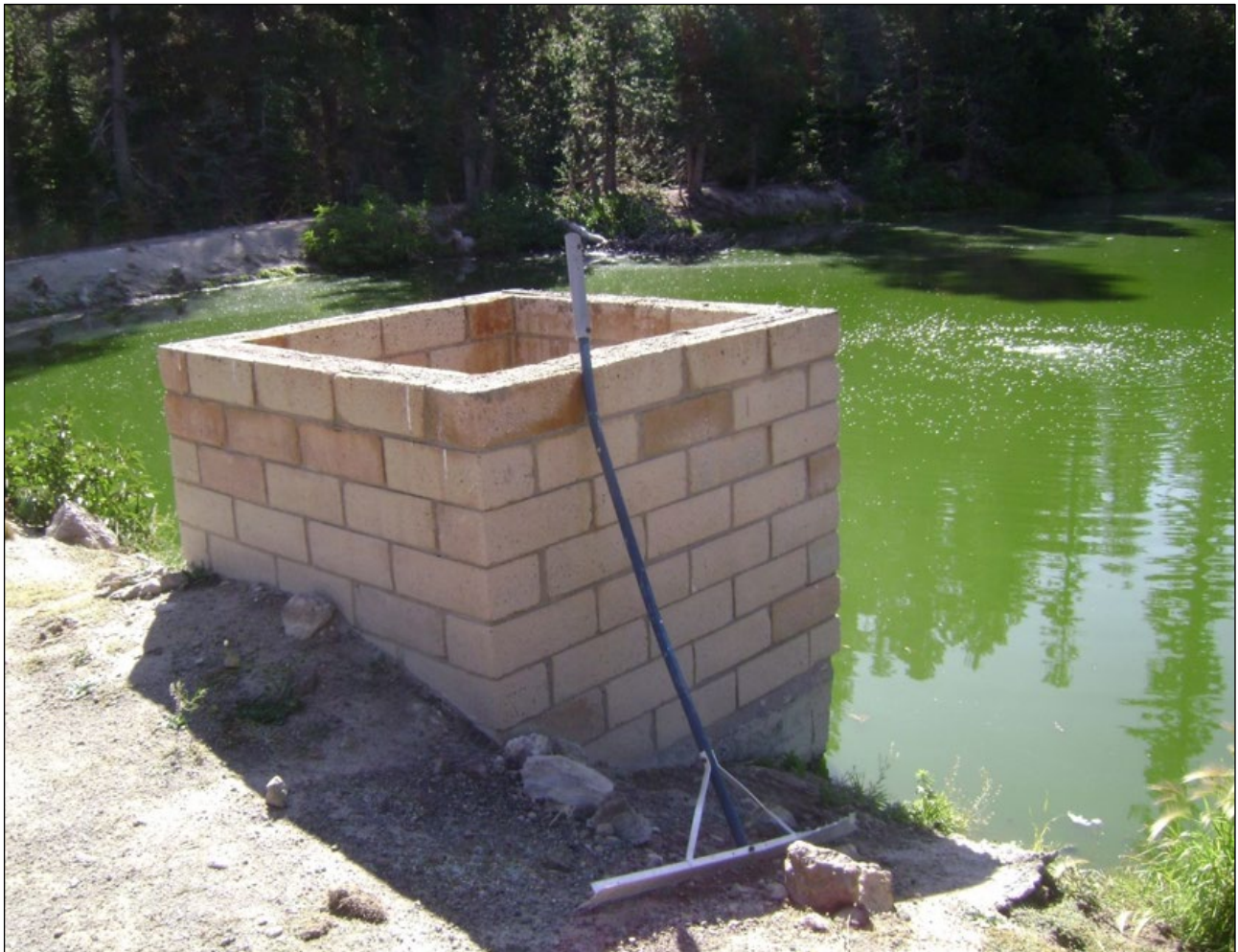
Figure 9.2 – MMSA raw sewage disposal pond. Green color indicates excessive algae growth caused, in part, by elevated nutrients in the effluent. Floating sewage debris is removed by hand using the rake shown, collected, and disposed offsite.
