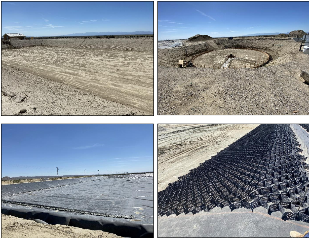
Figure 6.1 – Rosamond Water Reclamation Plant, May 13, 2020. Top Left: Excavation area of Biolac® aeration pond. Top Right: Excavation area for circular secondary clarifier. Bottom Left: Liner installation of emergency storage pond. Bottom Right: Geoweb® geocell installation on percolation pond side-slopes.
