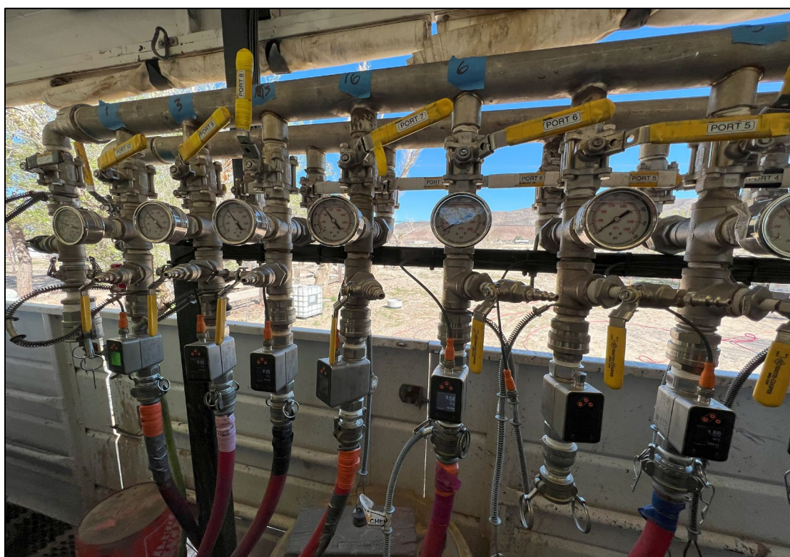
Photo 5.3: The pressure and flow manifold. Up to 10 borings were injected simultaneously.
