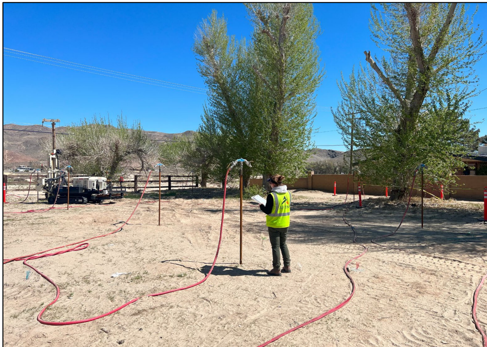
Photo 5.7: Field technician checking connections and making note of injection operations in the “garden area.” Photo facing northeast.
