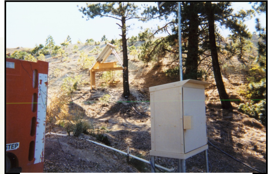
USGS Stage and Flow Monitoring
