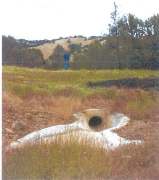
Photograph B-40: Storm water runoff outlet piping from upper mine workings area.
