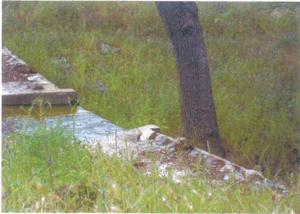
Photograph B-37: Weir on My Creek below retention pond (sample location SW-13).
