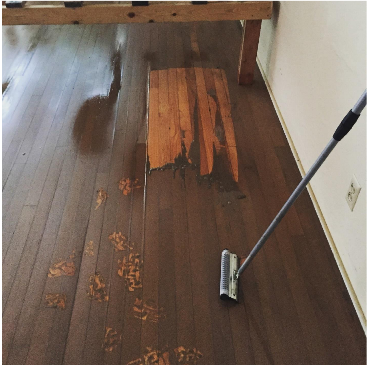
Figure 1: Evidence of flooding on January 17, 2016. The dark is sediment left by the flood. The lighter color is a section of flooring after I cleaned off the sediment. Photo by Kristi Wrigley.
