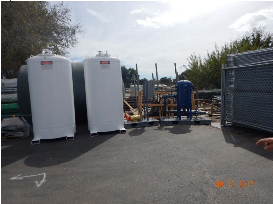
Photo 6. Treatment system components staged for future installation. According to Facility staff, the system installation will begin once building permits are received.
