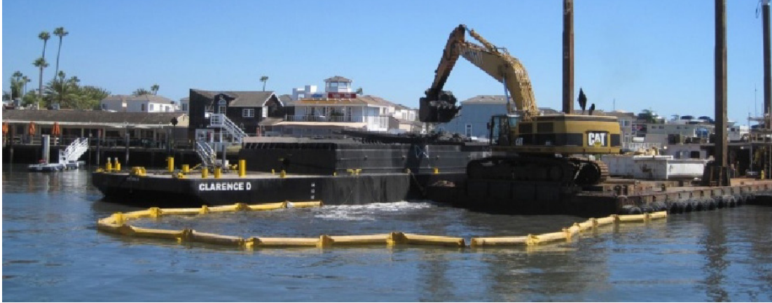
Rhine Channel Remediation Project; crane using clamshell bucket. Photo by: Chris Miller, City of Newport Beach.
