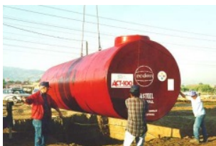
Underground storage tank
