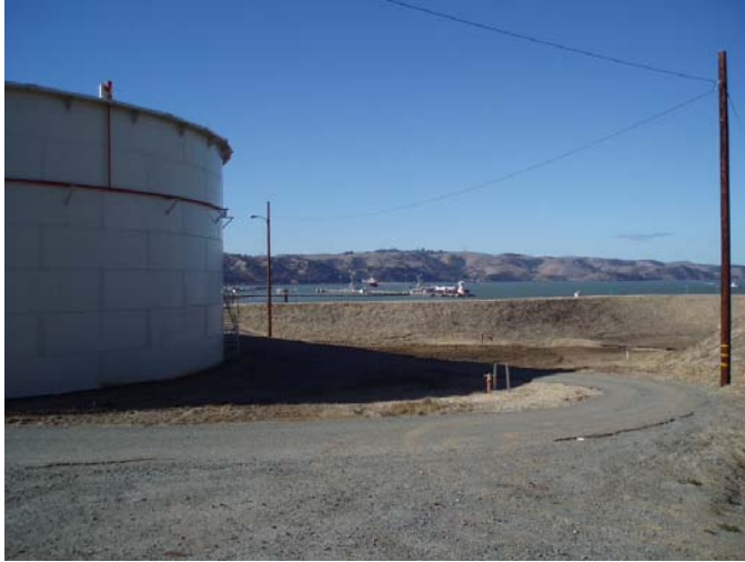
Figure 1: Past MTBE storage resulted in leakage from this tank and/or underground piping
