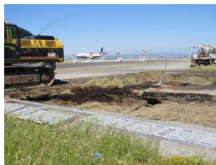
Photo 2. Excavation Pits with Dark Patches Showing Jet Fuel
