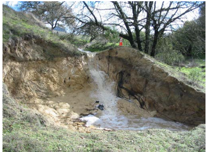
December 2002 – Uncontrolled runoff from construction site causes large scale erosion, continuing to fill in pond and riparian area.
