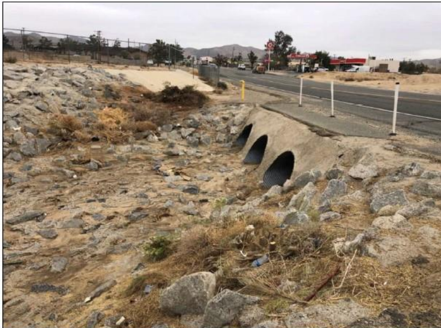
Figure 8. Photograph of impacted area PM 0.3, eastside.
