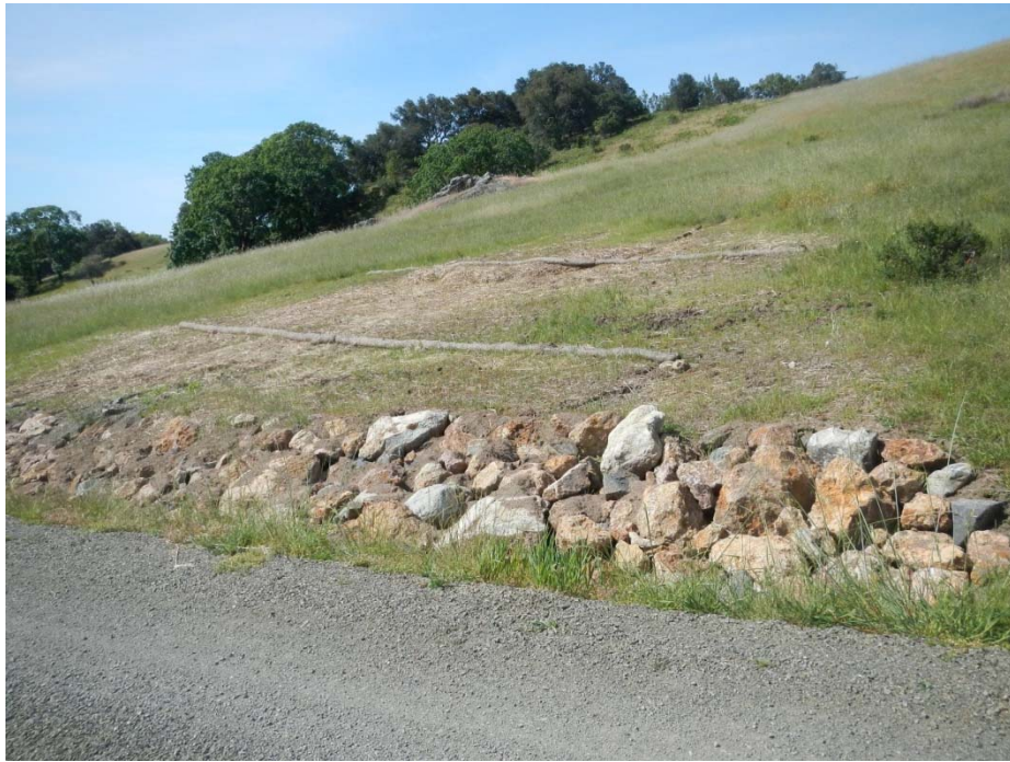
PWA Site 7.2 landslide (May 2014)
