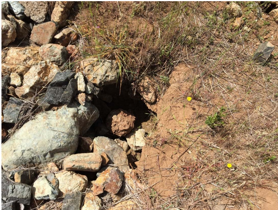
PWA Site #8.1 Grade Control Structure Headcut (May 2015)
