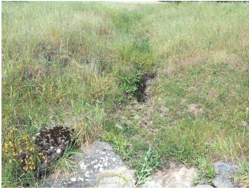
Headcut above PWA Site #6.2, below PWA Site #8.1 (May 2015)
