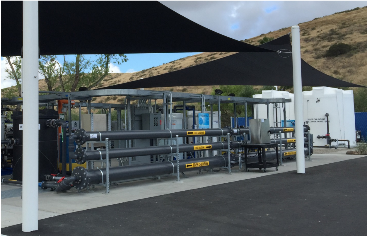
Padre Dam Advanced Water Purification Demonstration Facility
