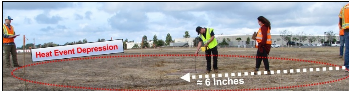
Figure 4: Inspection photograph of the heat depression within the Unit 3 cover.
