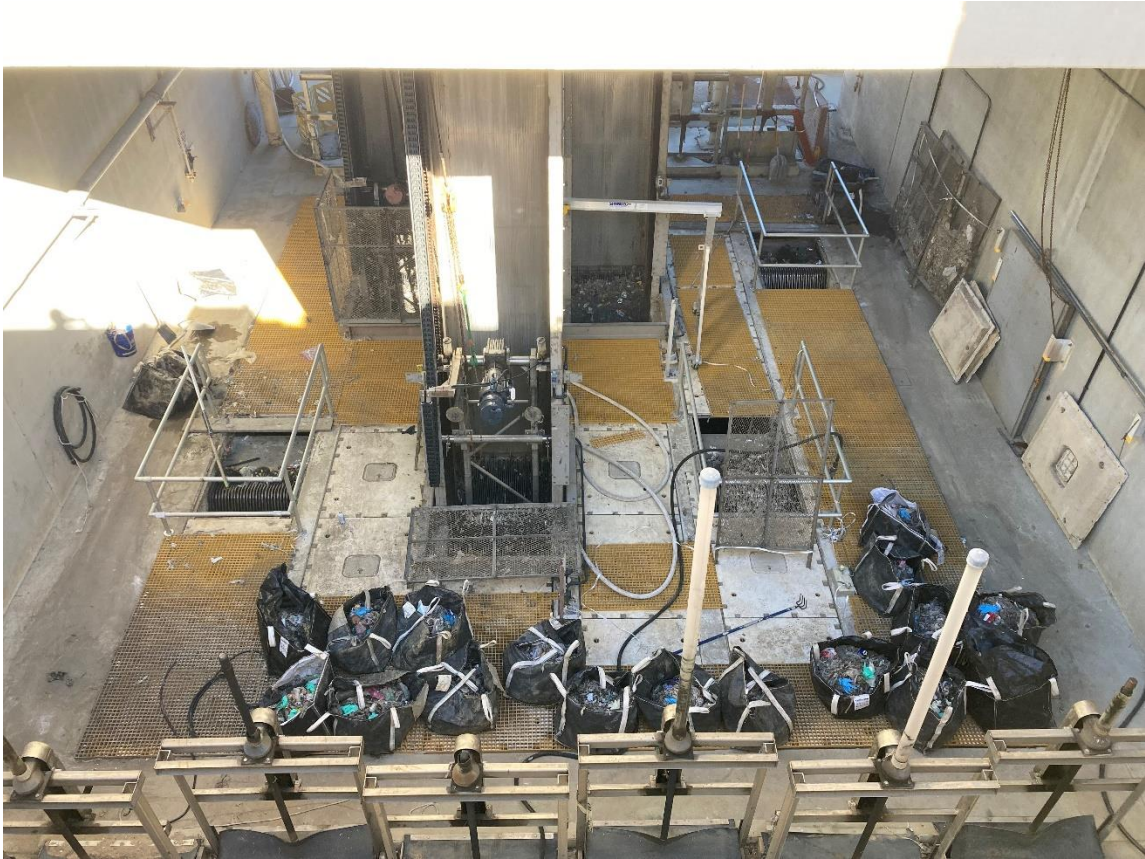
Figure 2: Bar Racks: Note bags of hand pulled rags from 5 days of manual operation (DWG 11-22-23).
