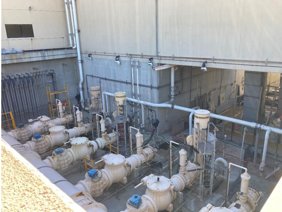
Figure 3: Three ITP Influent Pumps in Operation (DWG 11-22-23).
