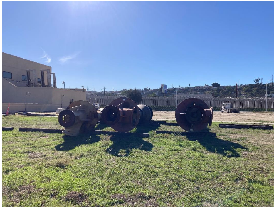
Figure 4: Three failed influent pumps pulled for replacement (DWG 11-22-23).
