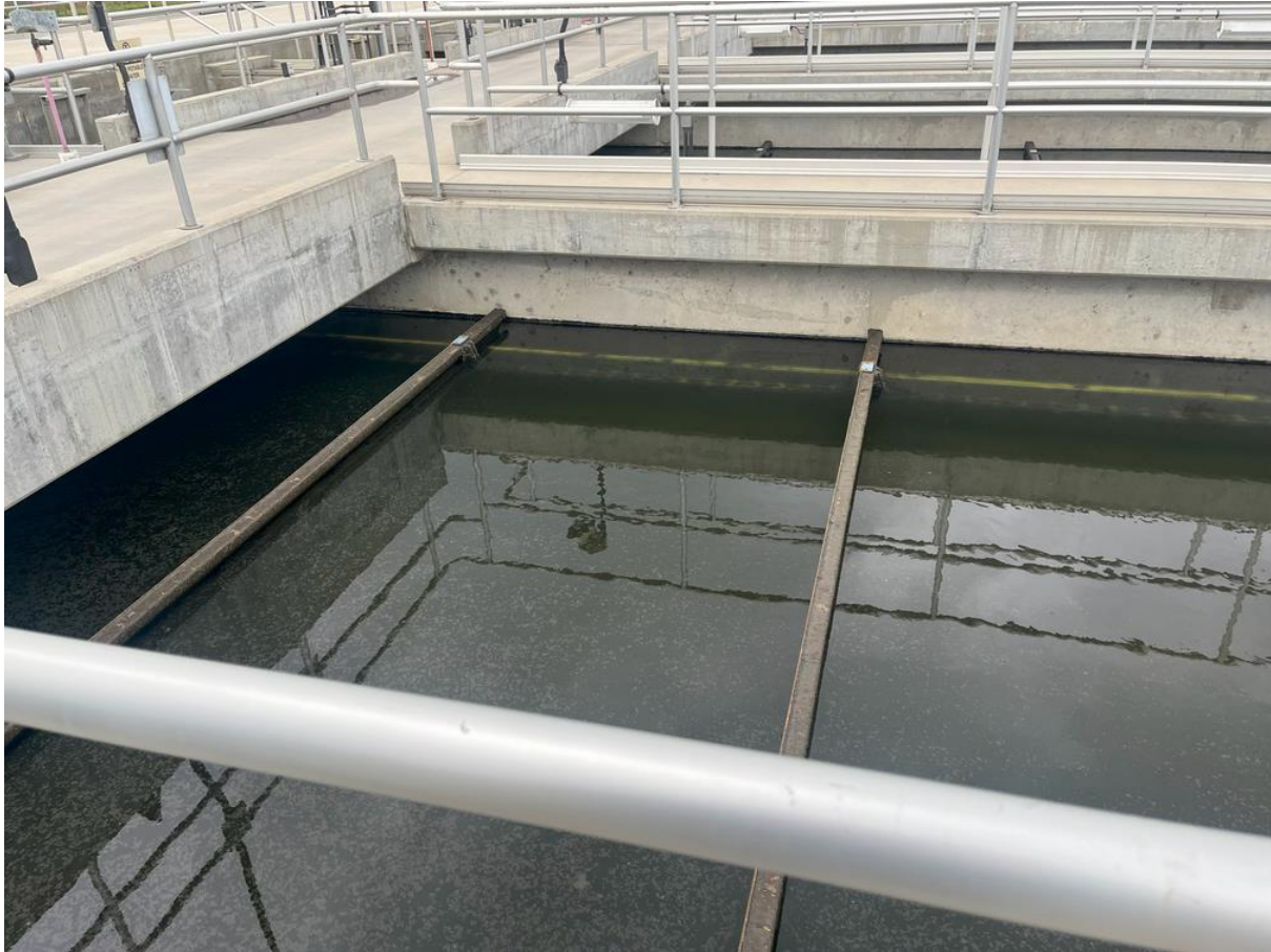
Figure 2: Secondary settling tank. (MC 01/10/2024)
