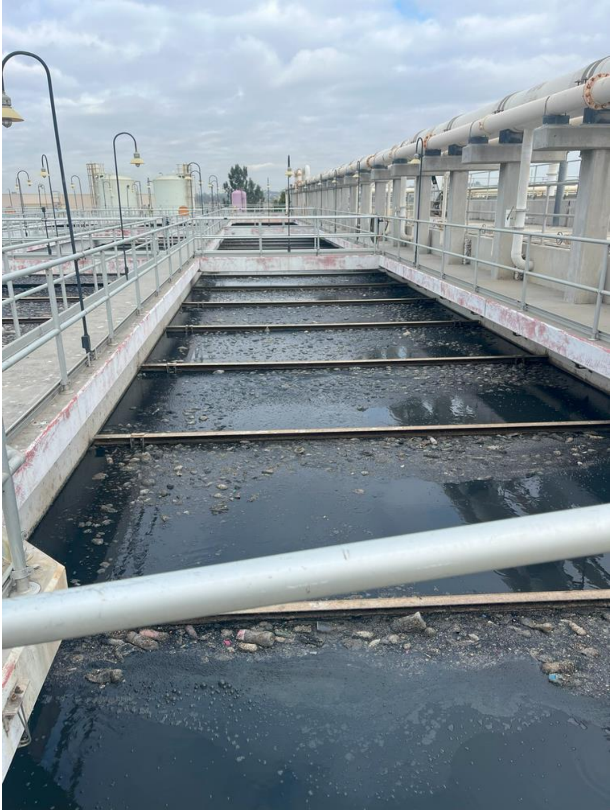
Figure 7: PST No. 1 is inoperable. (MC 01/10/2024)
