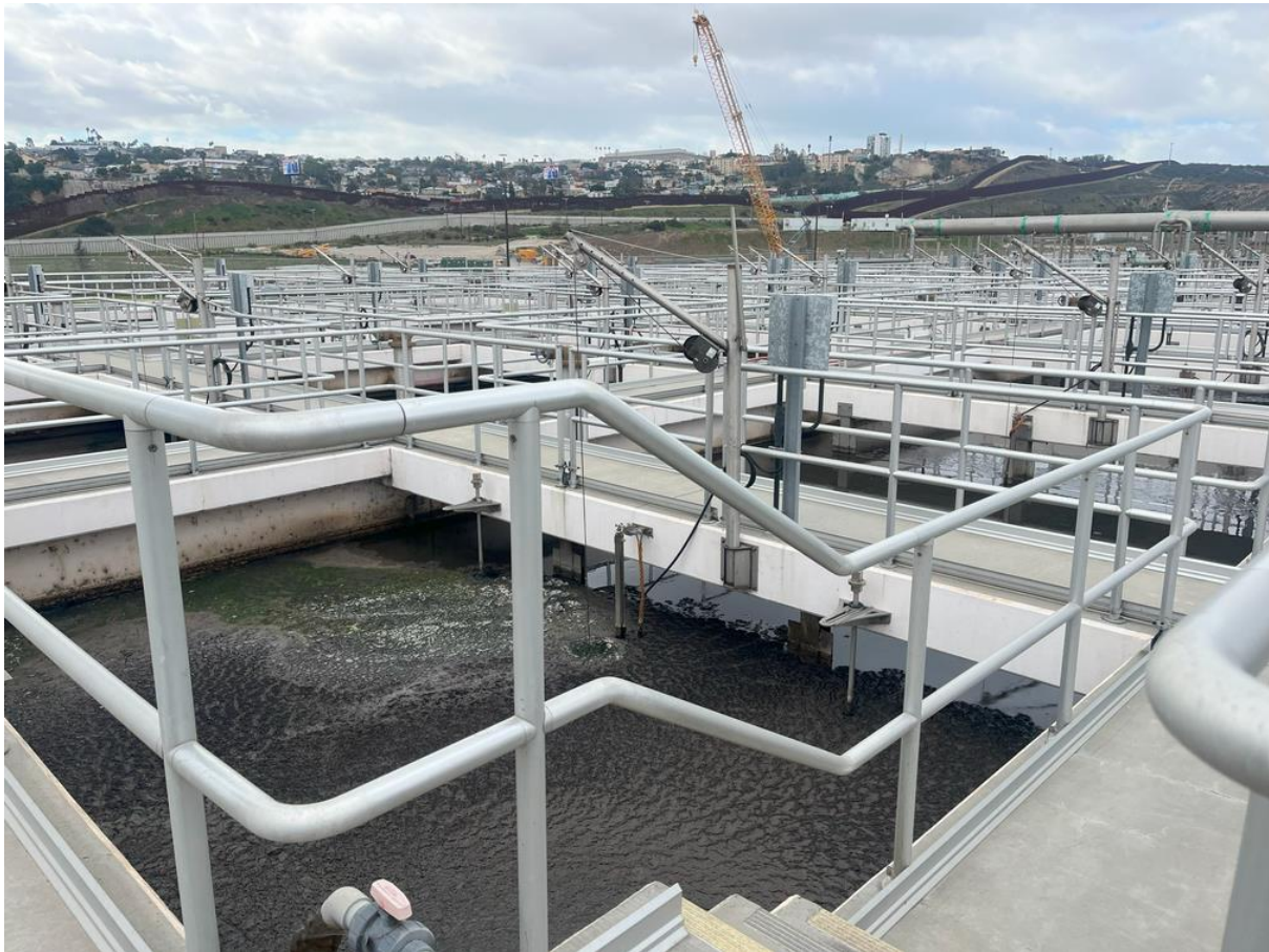
Figure 8: Secondary aeration tank. (MC 01/10/2024)
