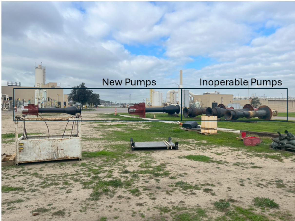
Figure 3: Two new influent pumps on the left. Three inoperable influent pumps on the right that have been removed for replacement. (MC 01/10/2024)
