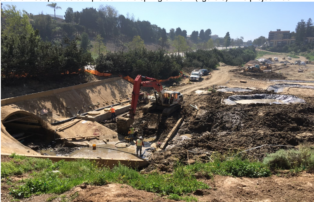
Figure 9: Big Canyon Nature Park Restoration Project's Selenium Diversion Project and Creek Bypass Construction
