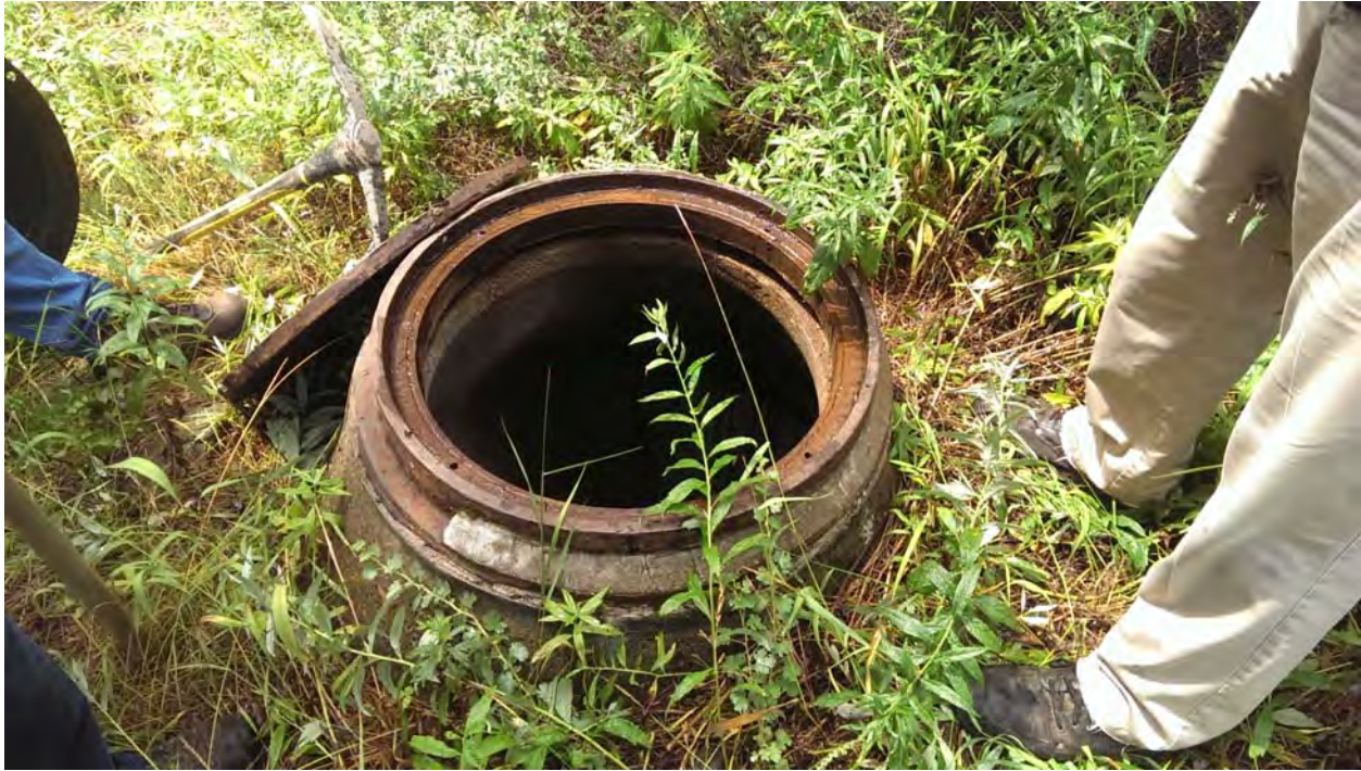
Spring well with cover removed.
