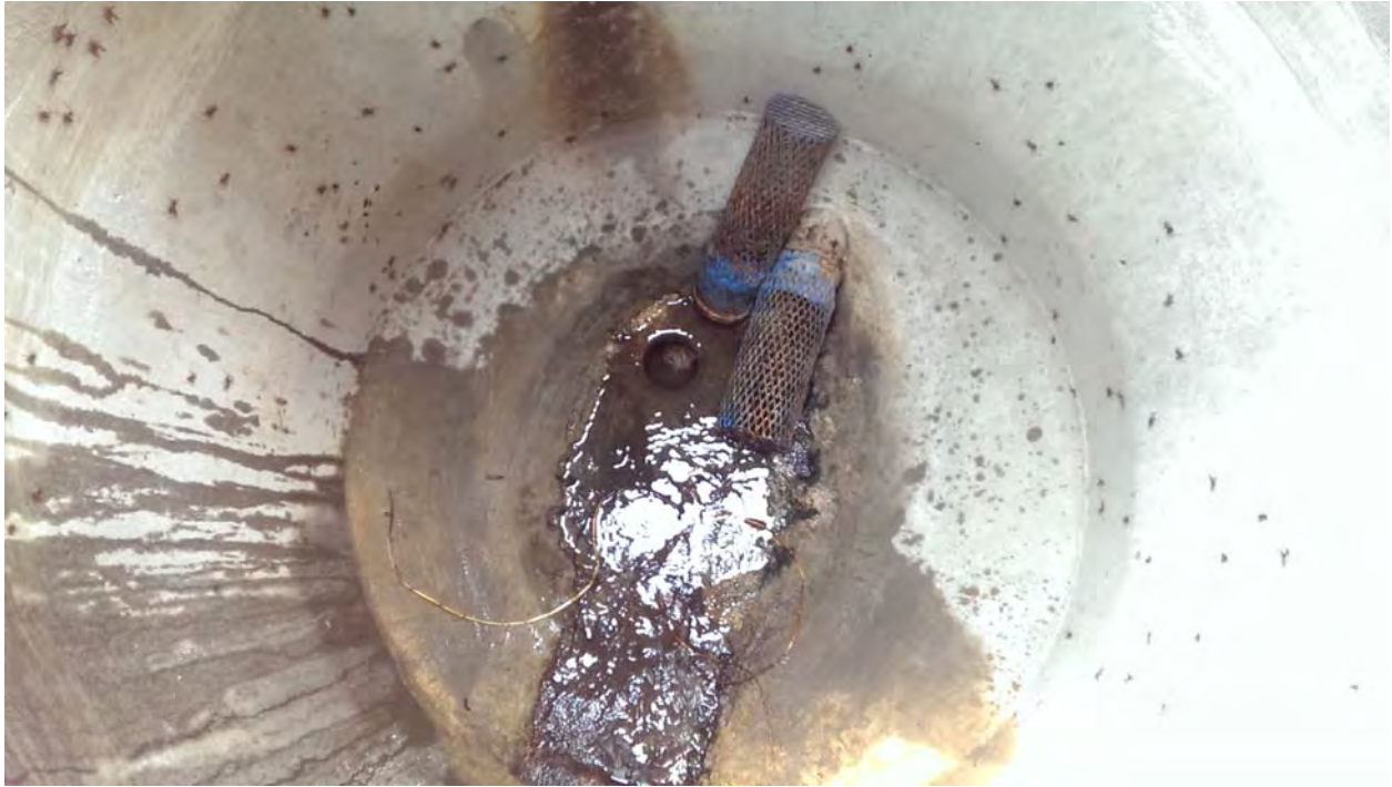
Vertical bypass pipe with cap removed so that all water is bypassed, due to cricket infestation.
