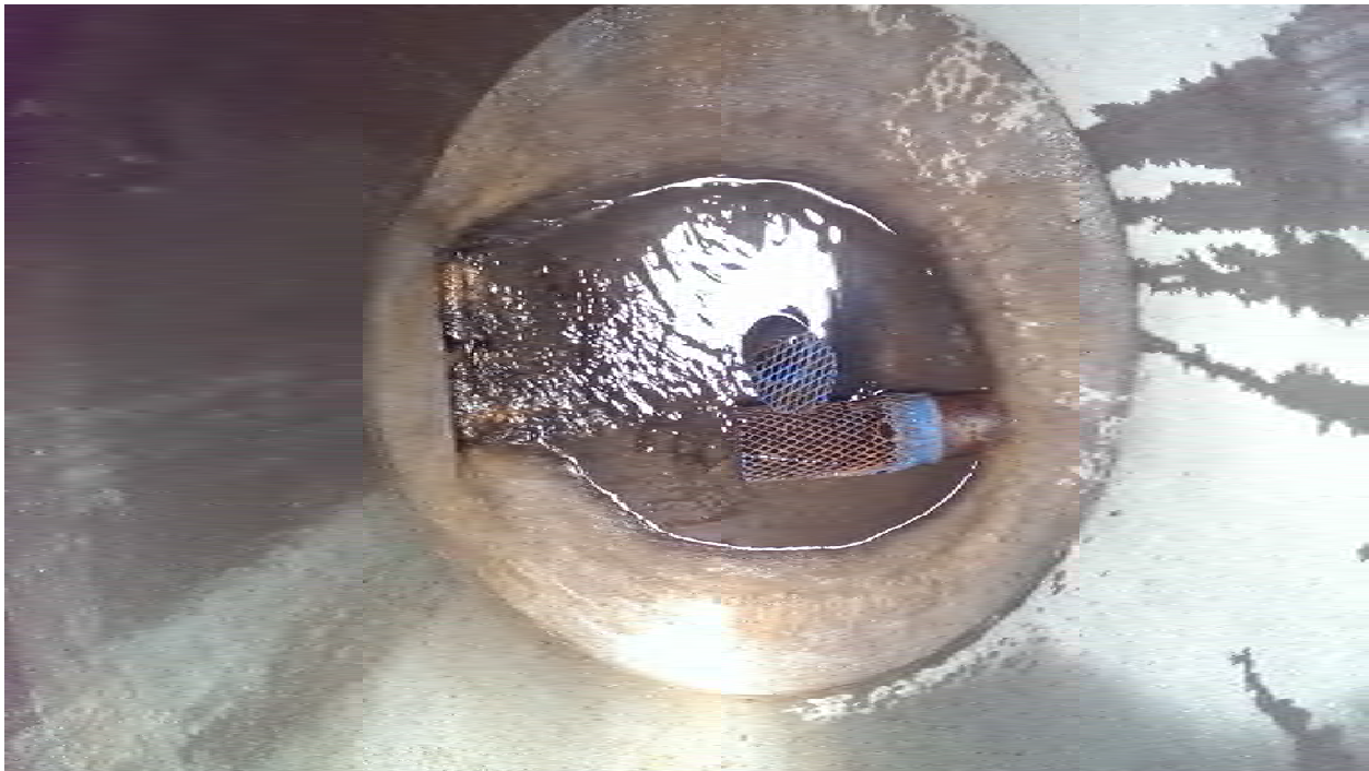
Inside spring well. Perforated horizontal pipe collects sub-surface water and enters the well from the left side. Vertical pipe at center bypasses flow when water level exceeds 4-6 inches. Horizontal pipe at right diverts water to collection system.
