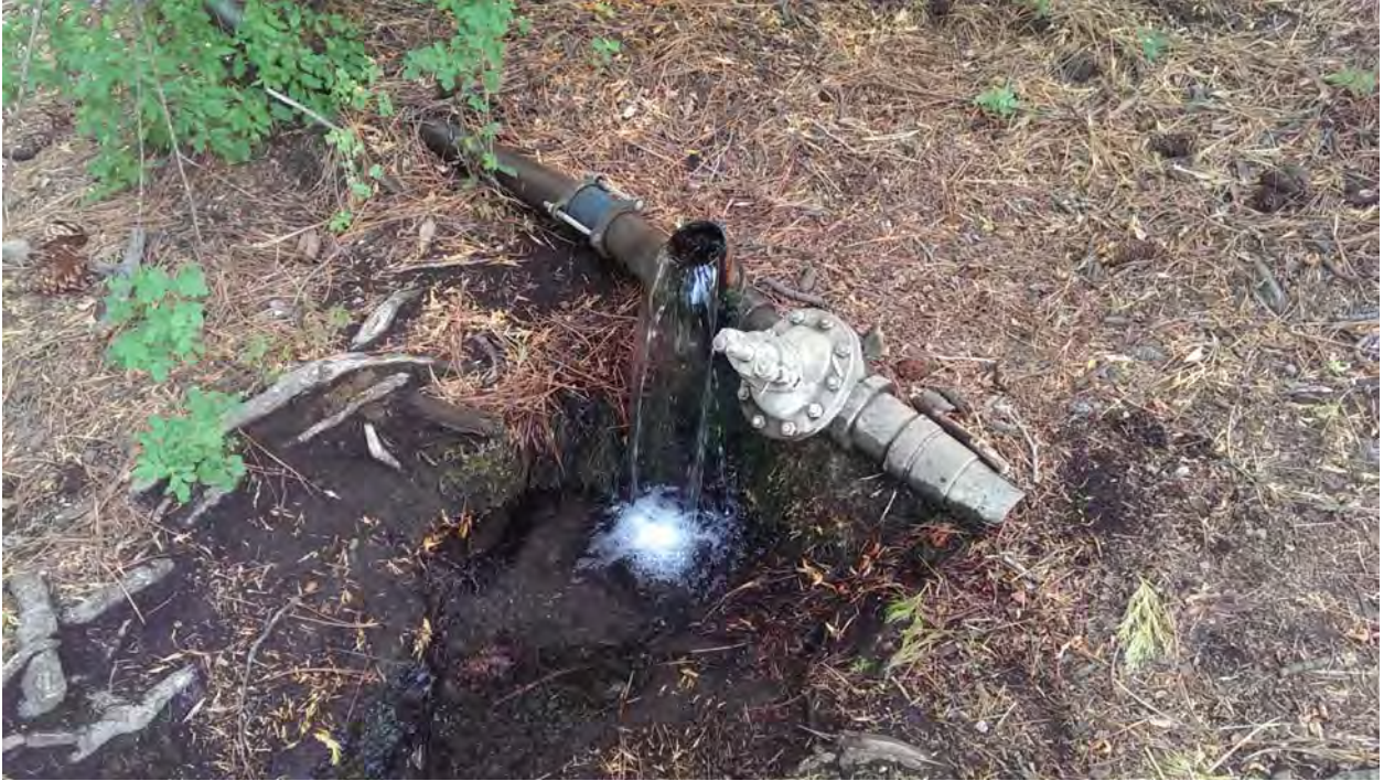
Discharge of water diverted at Pre-1914 well. Pipe disconnected from distribution system (at right).
