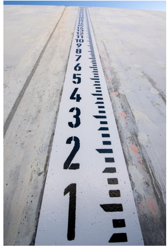
Figure 2. Several staff gauges have been installed on the inside walls of the newly constructed Lake Oroville main spillway in Butte County.
