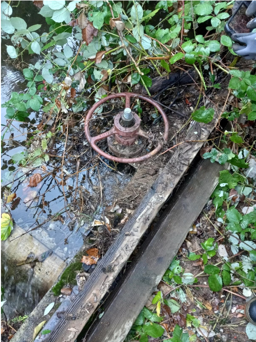
Photo 4 Penstock intake valve locked in the open position.
