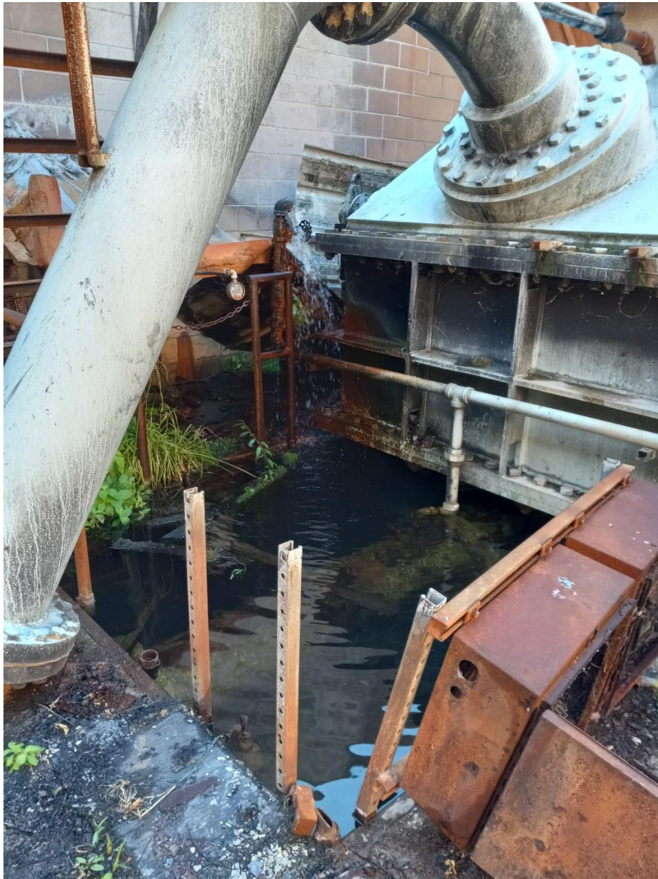
Photo 6 Maintenance pit full of water and penstock actively leaking.
