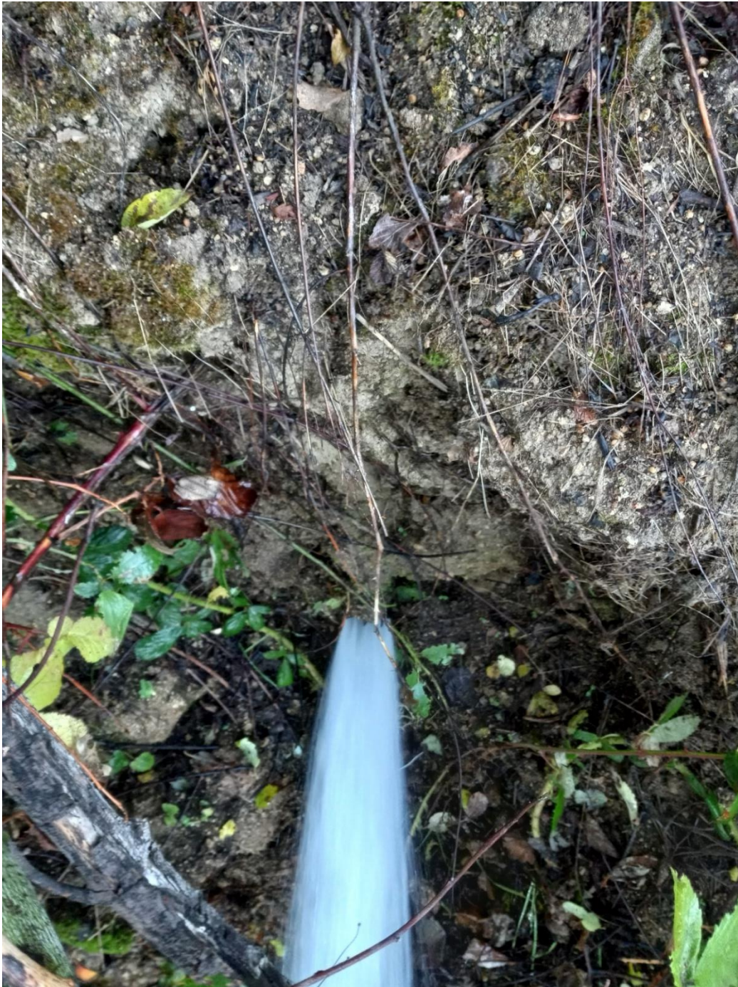
Photo 1 Failed pressure release system and erosion on downhill side of the Diversion Dam access road. Water discharges are associated with ongoing penstock diversions.
