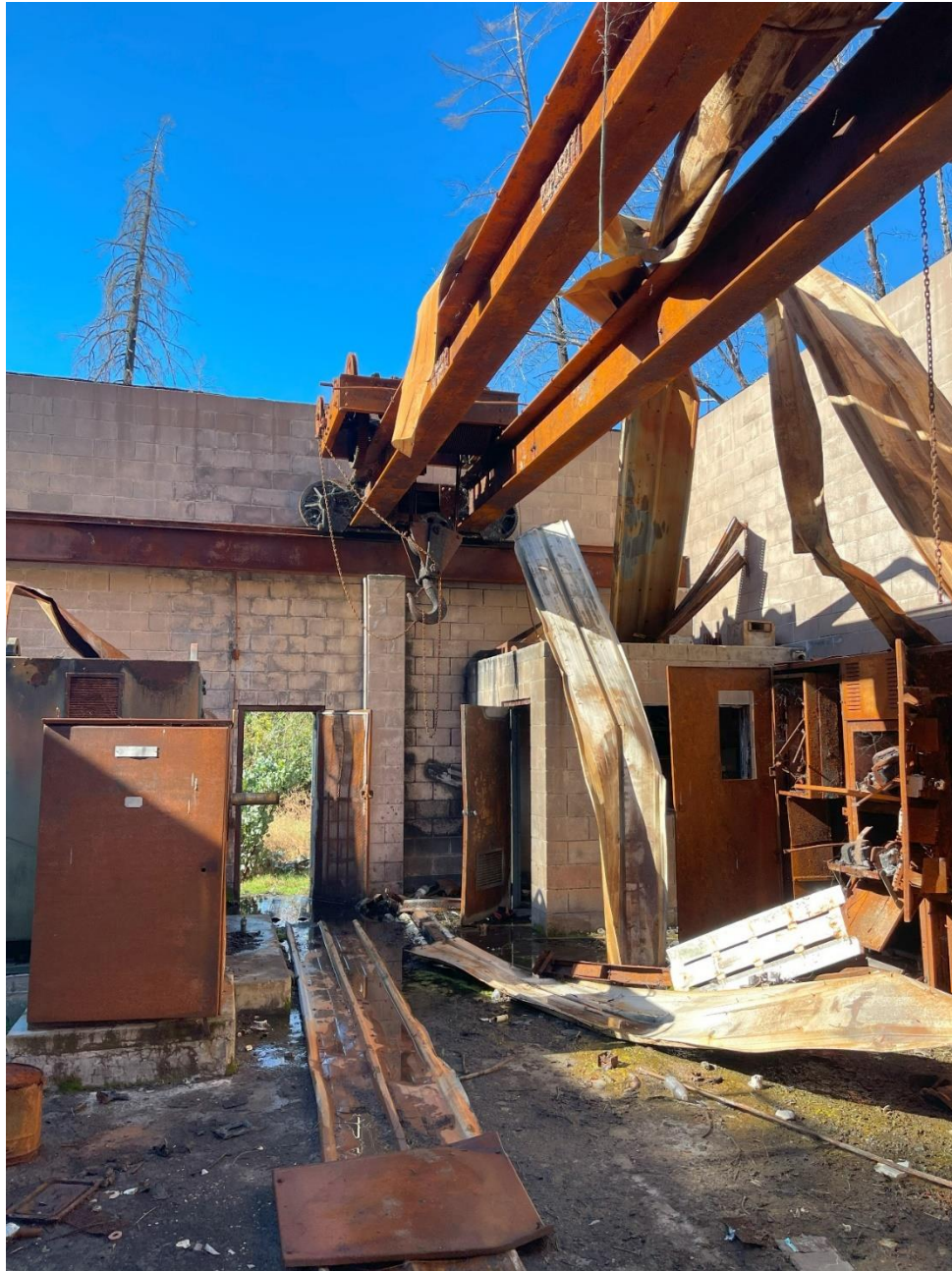
Photo 5 Powerhouse operational material left in place since the 2017 Ponderosa Fire.
