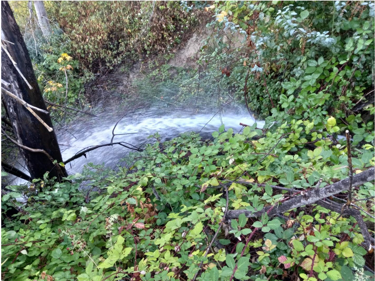
Photo 2 Failed pressure release system and erosion on downhill side of the Diversion Dam access road. Hillslope instability shown in the background.
