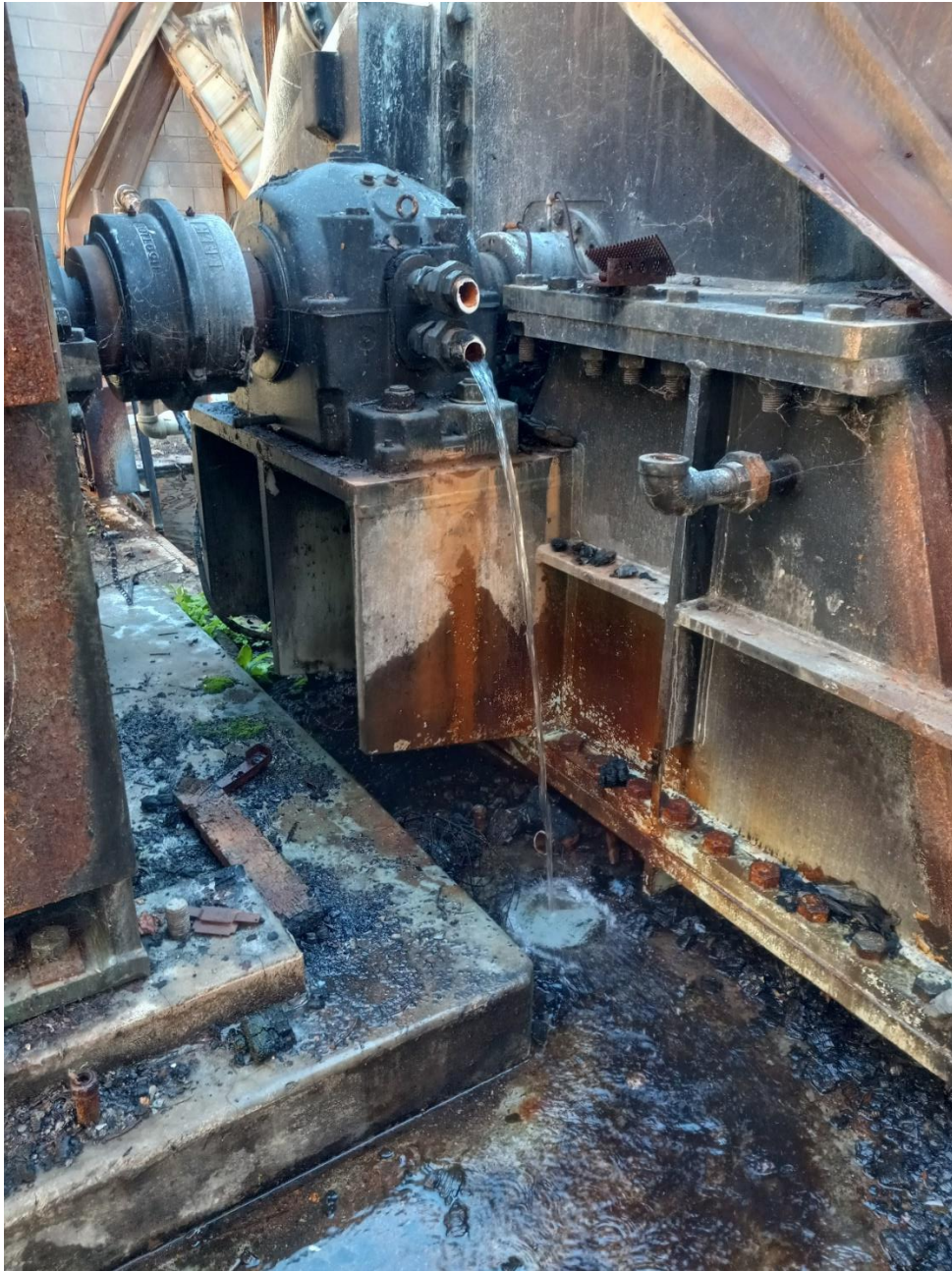
Photo 7 Water actively leaking from power generation equipment.
