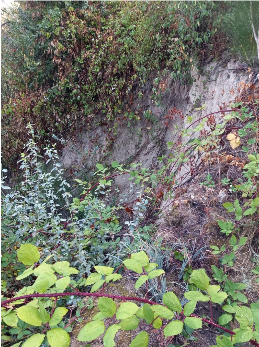
Photo 3 Hillslope instability near penstock leak on downhill side of the road.
