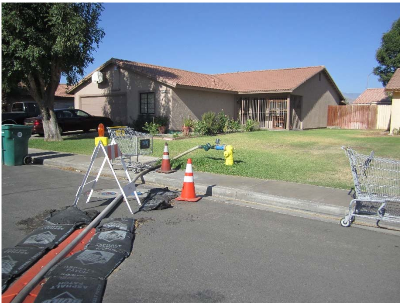
Image: 2013 temporary intertie with IWA.
