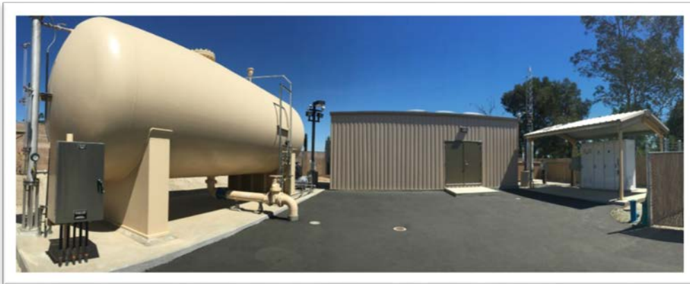
Part of the consolidation effort included new water infrastructure, such as a new water pump station.
