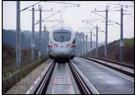
Typical Overhead Catenary
