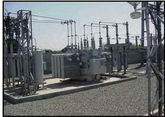
Typical Electric Substation
