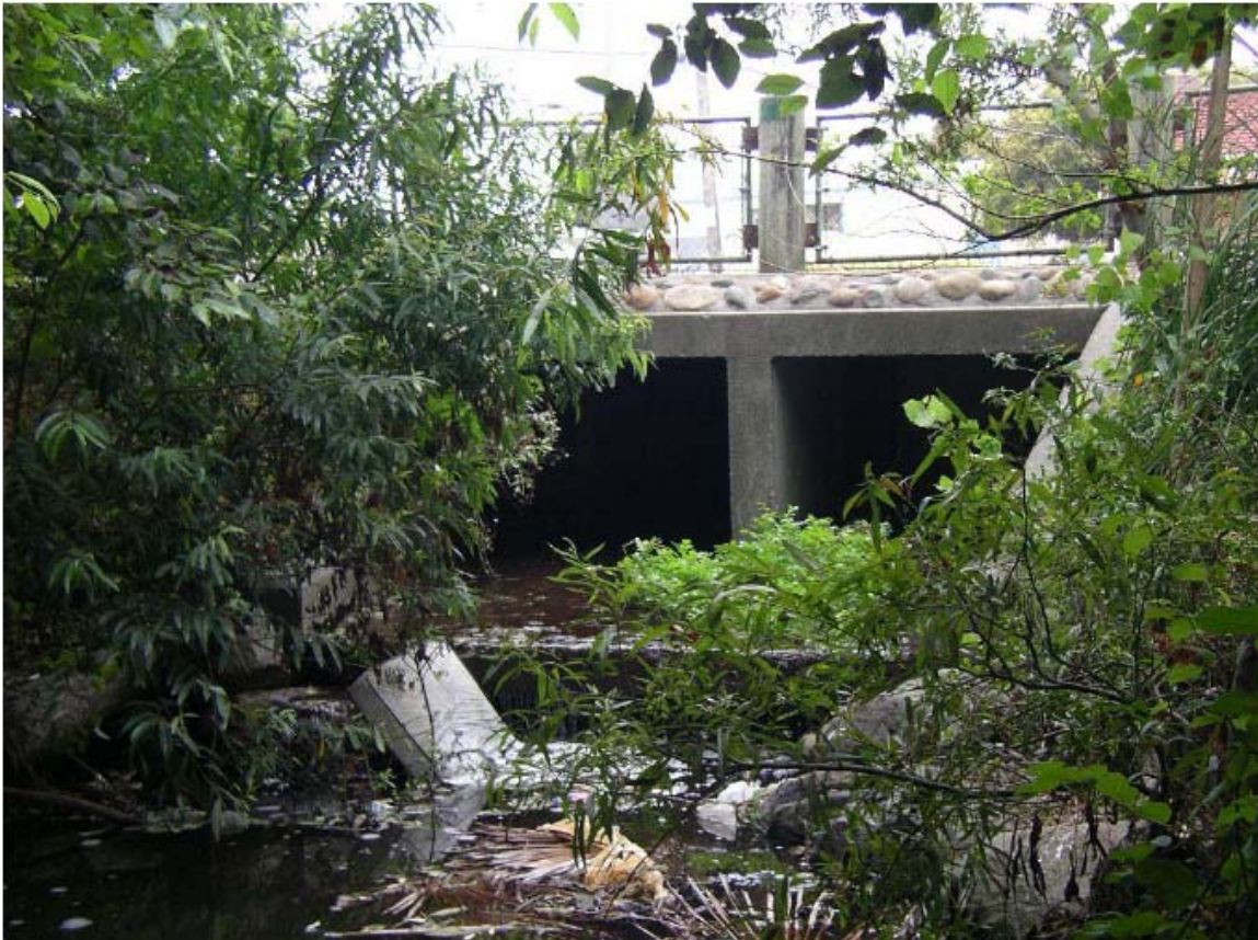
Figure 10: View looking upstream from Booker T. Anderson Park trash survey site (BAX030), showing dumped mattress and low fence above culvert at street crossing, upstream of park. Photo by Steve Moore, August 23, 2005.
