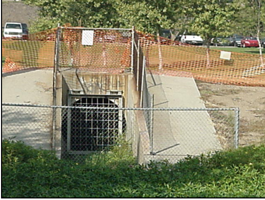
Figure 6.3-1. Machado Lake trash screen.
