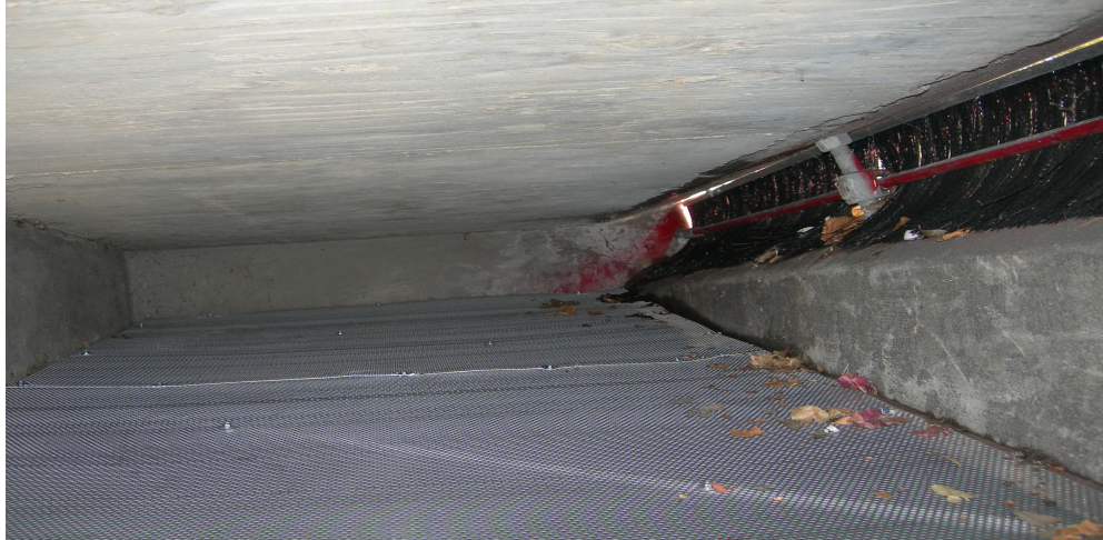
Figure 5-6 Metal mesh installed within the catch basin to collect trash not retained by the brush at the inlet.
