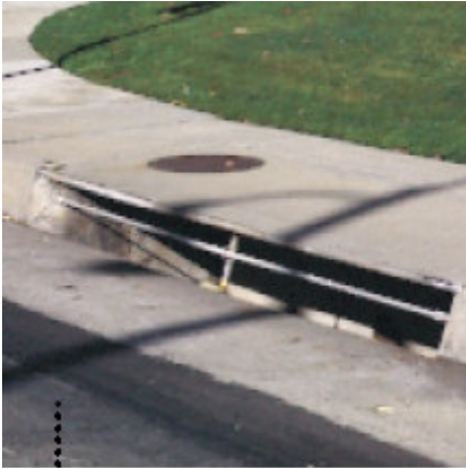
Catch Basins are the major entry points to the storm drain system
