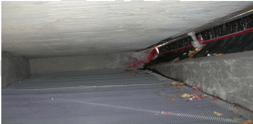
Figure 6-6 Metal mesh installed within the catch basin to collect trash not retained by the brush at the inlet.
