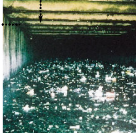
Underground drains carry runoff into larger channels such as this
