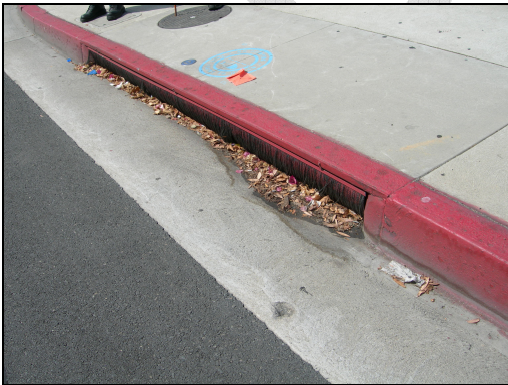
Figure 8-2. City of Glendale, catch basin brush insert
