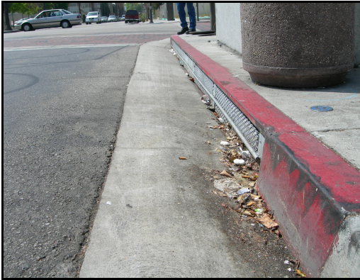
Figure 8-1. City of Glendale, catch basin insert
