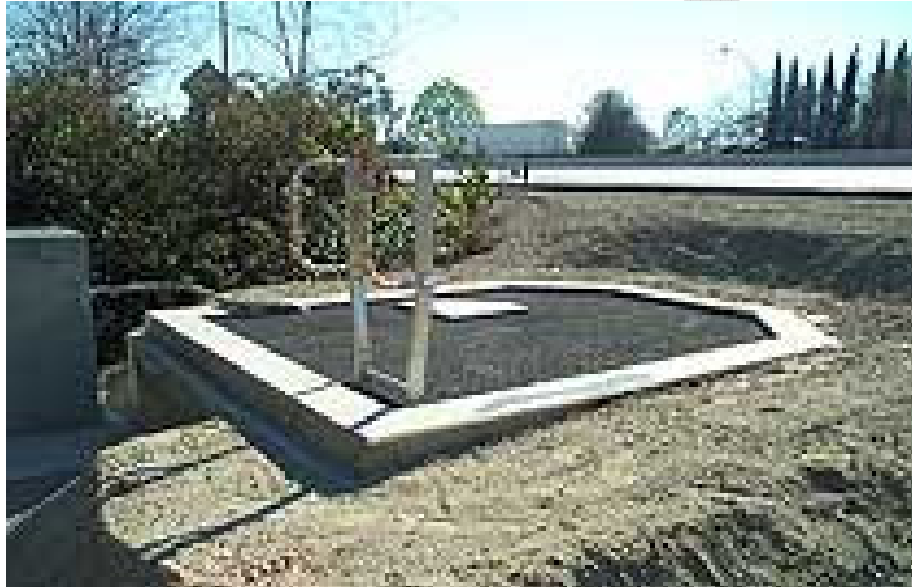
Figure 7.3-4. Location with GSRD Installation.
