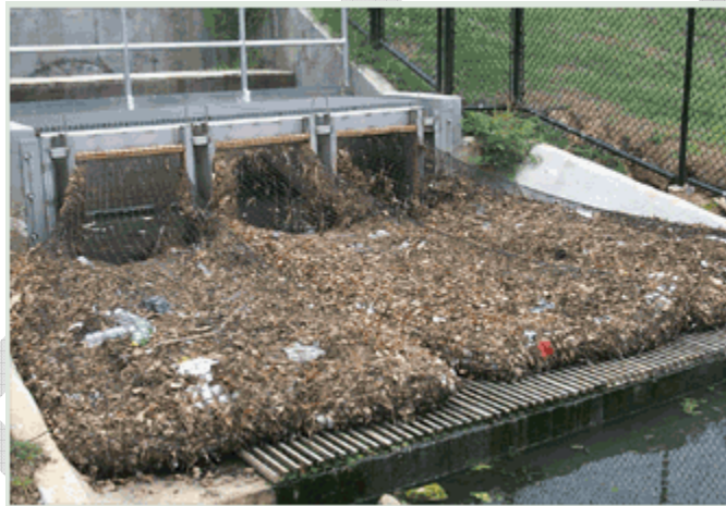
Figure 7.3-3. Picture of end-of-pipe trash net containing trash.
