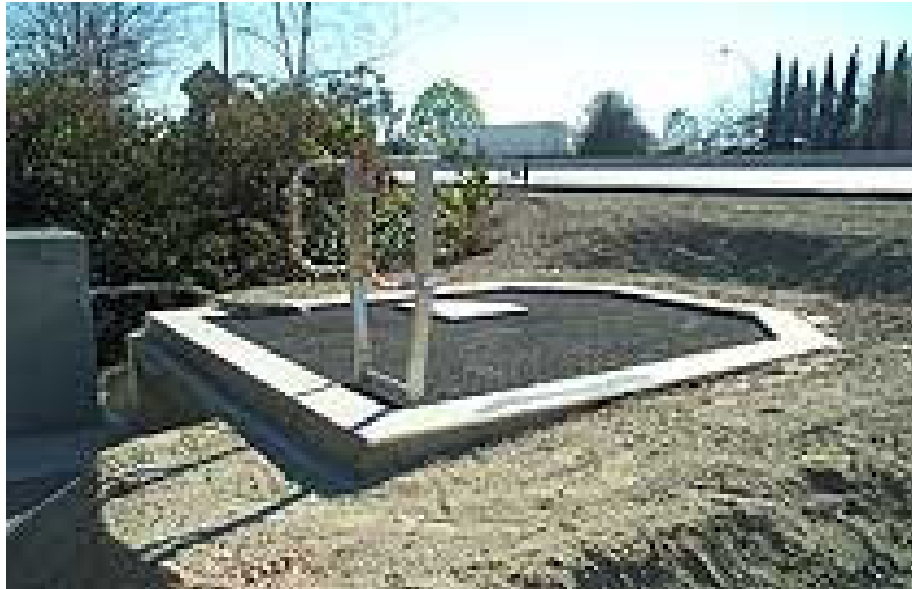
Figure 6.4-4. Location with GSRD Installation.
