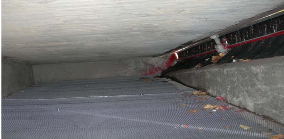
Figure 5-6 Metal mesh installed within the catch basin to collect trash not retained by the brush at the inlet.
