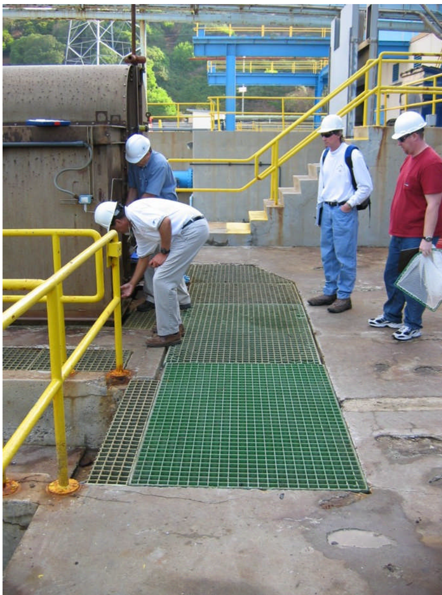
Figure B4-2. Units 3&4 traveling screen collection basket under central green grate.
