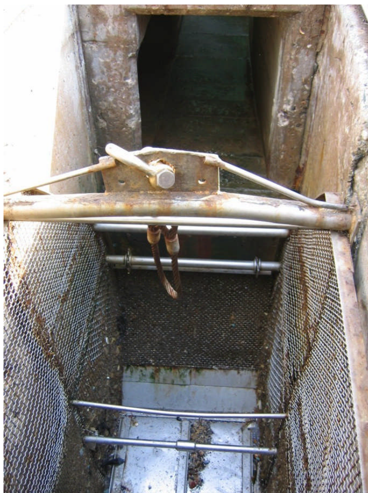
Figure B4-1. Units 1&2 traveling screen collection basket.
