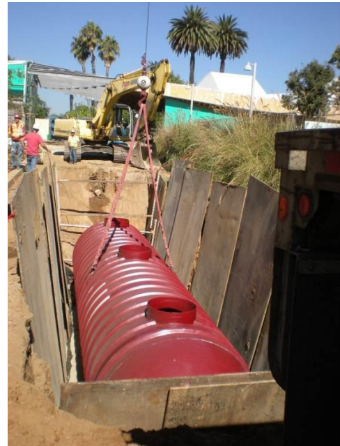
A subsurface storage tank and treatment system being installed (source: Neal Shapiro, City of Santa Monica)
