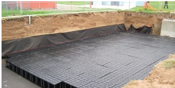
Subsurface Infiltration Gallery
