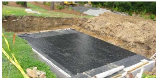
Subsurface Detention Gallery
