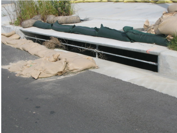
Photo 11. Unprotected storm drain inlet.
