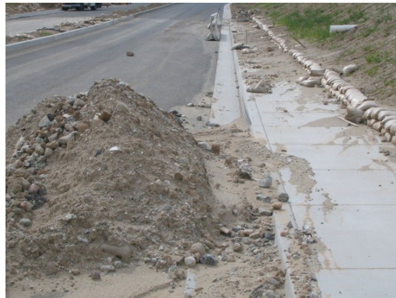
Photo 17. Unprotected stockpile in drainageway.
