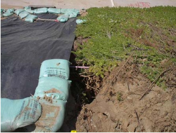
Photo 3. Slope failure at edge of visquine.
