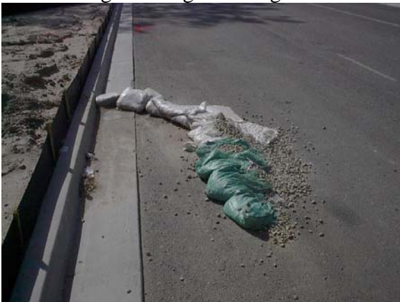
Photo 10. Gravel bag berm with broken gravel bags.
