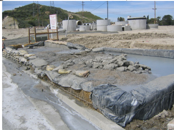
Photo 20: Failed concrete washout.
