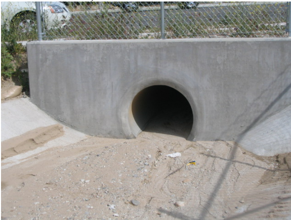
Photo 1. Failure to clean and maintain culvert.
