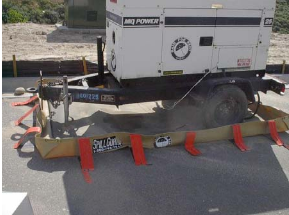
Photo 18. Secondary containment under generator.
