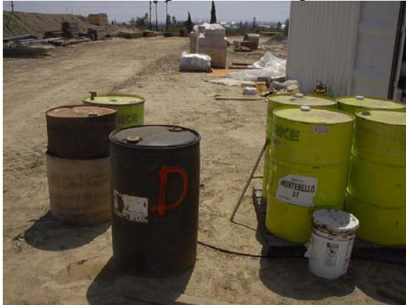
Photo 15. Improper storage of drums without secondary containment or overhead cover.
