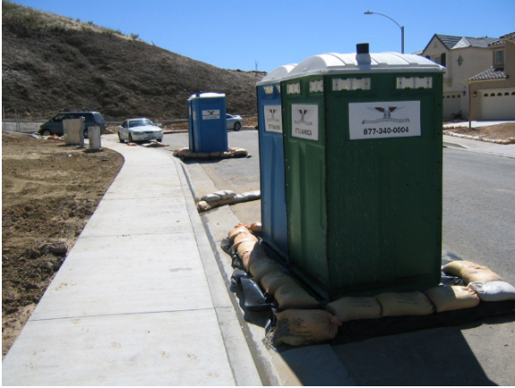
Photo 21. Secondary containment around portable toilets.
