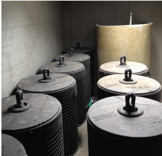
Figure 5: Contech MFS filter cartridges in underground concrete vault at SR431. Float valve is behind fiberglass shield. An outflow pipe runs underneath each row of cartridges.
