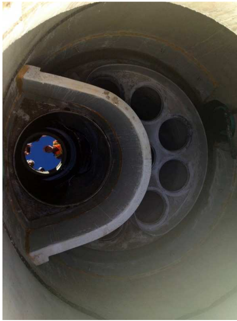
Figure 3: View looking down on Imbrium Jellyfish membrane filtration cartridges installed in concrete vault at SR431.
