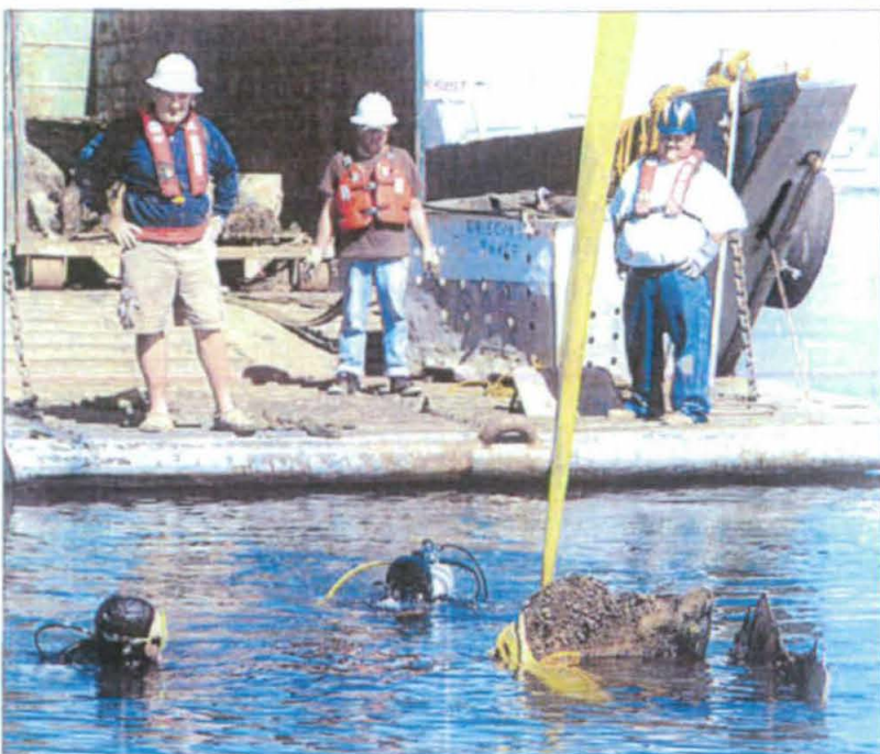
More Cleanup — San Diego Bay's old A-8 public anchorage was shut down in 2008, leaving behind sunken vessels and marine debris. While more than 700 pieces of debris and 75 boats were removed by 2010, recent sonar imaging of the anchorage and its surroundings identified 11 vessels and 945 items on the bottom still in need of removal.
