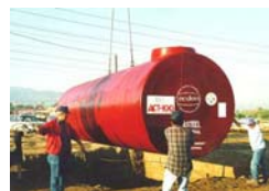
Underground storage tank
