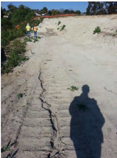
Photo 7: Signs of erosion on inactive areas of the site. Portion of the site without erosion or sediment control BMPs even though it has been inactive for more than 14 days (CGP requirement) which also exceeded the City's 10 day definition of inactive.
