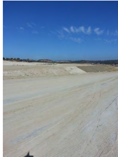
Photo 10 Partial erosion control present (i.e. straw blankets) on one large slope. Partial linear sediment controls on a part of the large slope in this photo. No erosion in conjunction with sediment controls present on other areas of site in this photo.
