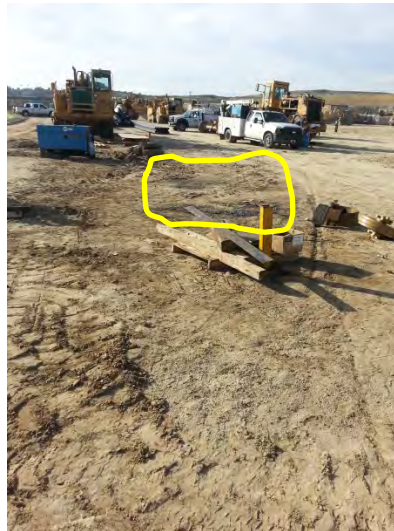
Photo 4: Leaks to the ground must be cleaned up immediately and disposed of leaked materials appropriately.
