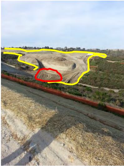
Photo 17 Large sediment basin (outlined in red) is the only BMP being relied upon to capture sediment and runoff from the approximately 45 acre portion of the site identified by the yellow line. At the time of this inspection this basin had not been designed in accordance with CASQA guidelines. No erosion controls present.
