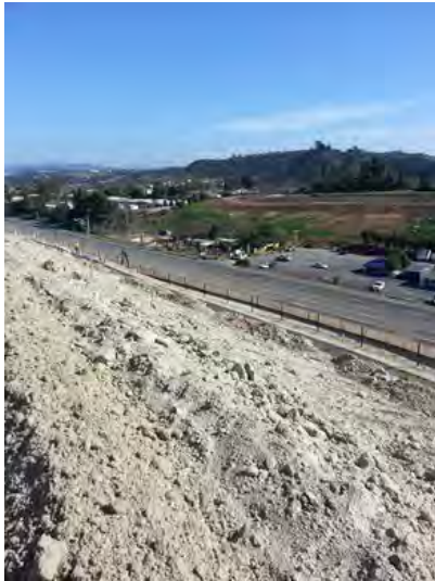
Photo 13 No erosion controls present on large slopes. No linear sediment controls on large slopes. No erosion in conjunction with sediment controls present on other areas of site.
