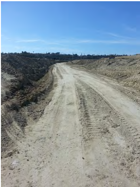
Photo 11 No erosion controls present on large slopes. No linear sediment controls on large slopes. No erosion in conjunction with sediment controls present on other areas of site.
