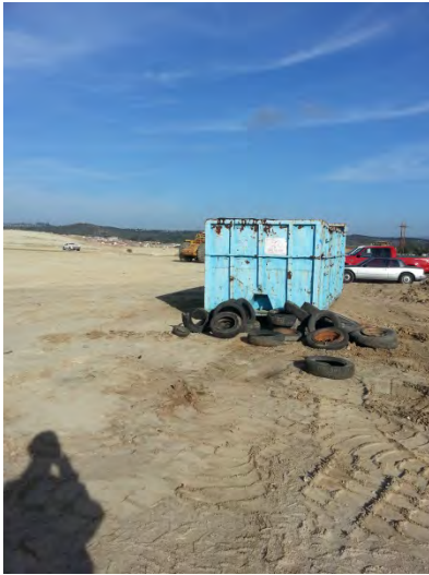
Photo 5: Stockpiled tires not contained and securely protected from rain. Waste bin not covered and no evidence of cover nearby indicating that the container is covered at the end of each workday.
