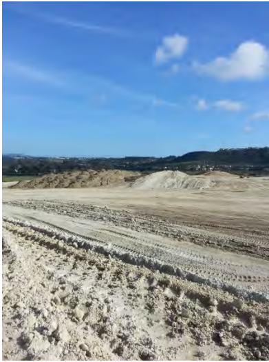
Photo 1: Loose soil stockpiles were not covered or bermed. Evidence supports stockpiles were not being used because there is no disturbance of pile.
