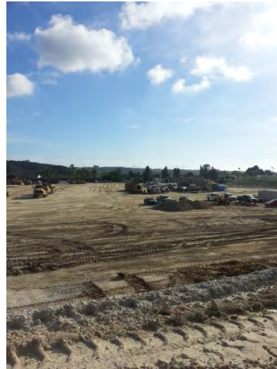
Photo 2: Loose piles of gravel were not covered or bermed. Evidence supports stockpiles were not being used because there is no disturbance of pile.
