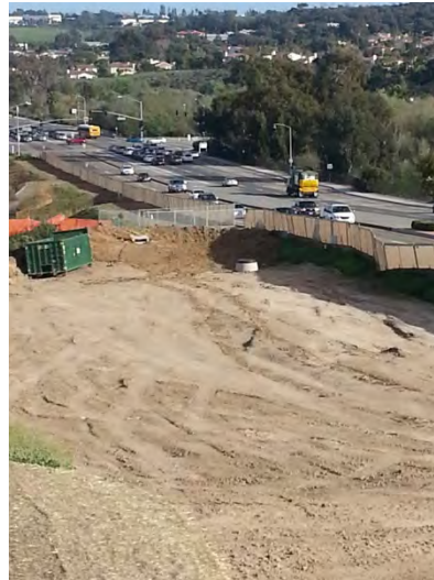
Photo 6: Waste bin not covered to provide protection from wind and rain. No evidence of cover nearby indicating that the container is covered at the end of each workday.
