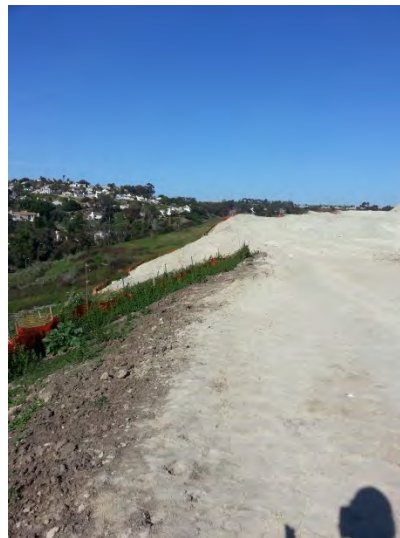
Photo 8: Large steep slopes along much of the perimeter of the site (this view is of the northern perimeter of the site parallel to Tamarack) without linear sediment controls or erosion controls. Portion of the site without erosion or sediment control BMPs even though it has been inactive for more than 14 days (CGP requirement) which also exceeded the City's 10 day definition of inactive. Silt fence is present at the toe of the slope that surrounds the perimeter of the site.
