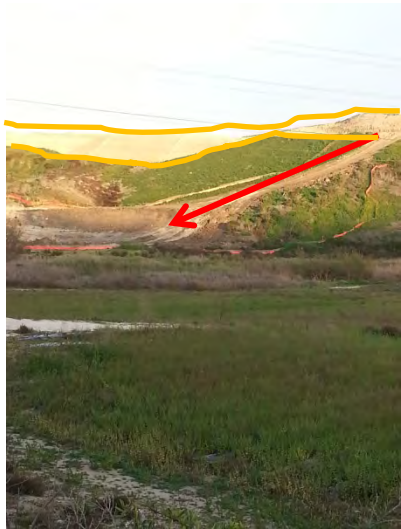
Photo 15 No erosion controls present on large steep slopes (red arrow). No linear sediment controls on large slopes steep slopes (outlined in orange). No erosion in conjunction with sediment controls present on either areas.
