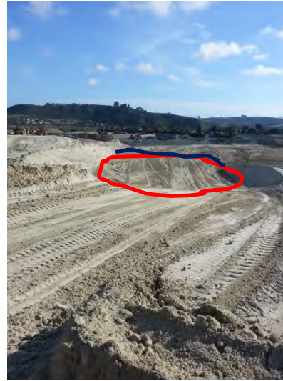
Photo 18 Large sediment basin (outlined in red) is the only BMP being relied upon to capture sediment and runoff from the surrounding area site shown in the photo. At the time of this inspection this basin had not been designed in accordance with CASQA guidelines. At the time of this inspection a berm to close off this basin (blue line) had not been constructed. No soil stabilization erosion controls are present. No linear sediment controls are in place on slopes. No erosion in conjunction with sediment controls present.
