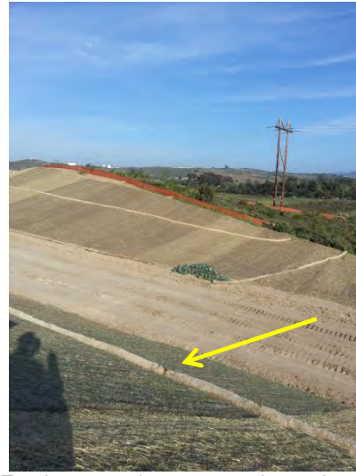
Photo 14 Erosion controls present only on slopes that have reached final grade. Linear sediment controls installed end to end and not overlapped per CASQA Construction BMP Handbooks. None of the fiber rolls on the site at the time of this inspection were installed with overlapping ends. It was unclear if the rolls were trenched in 4 inches.
