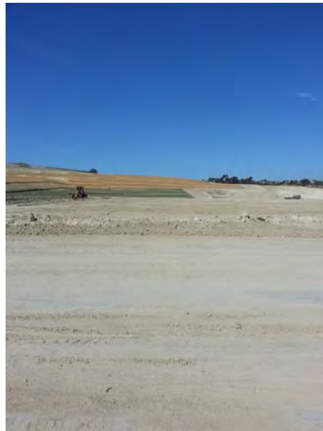
Photo 12 Erosion and sediment controls present only on those slopes that have reached final grade. No erosion in conjunction with sediment controls present on other areas of site.
