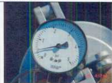
Diesel Fill, .5 psi
